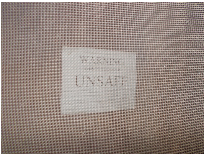
Photo 15 – Building 8, unsafe to enter building signage posted.
