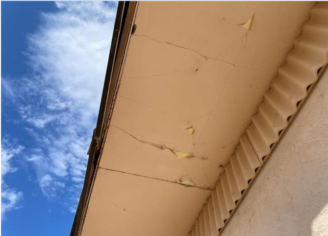
Figure 6 - Moisture movement into the deck assembly by exterior fascia and soffit paint repair and retrofit is necessary to attempt to eliminate moisture absorption by the gypsum and fiber formboards.
