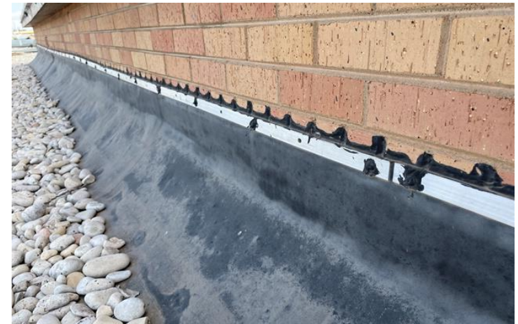
Figure 4 - Base flashing membrane does not appear to be the original membrane and has been improperly sealed to the exterior face of brick cladding. This condition may have contributed to moisture underlying the membrane even though the membrane does not appear to have been damaged
