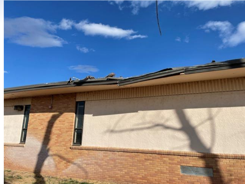
Figure 5 - Portion of the roof deck that has been damaged by falling tree limbs
