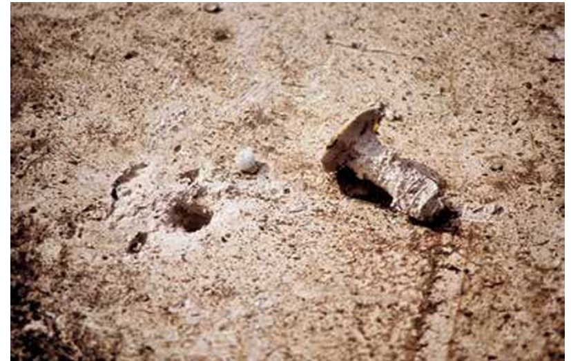
Figure 7 - Photograph of a gypsum deck NOT from this inspection that demonstrates lack of withdrawal resistance necessary to support a new roof due to prolonged moisture damage
