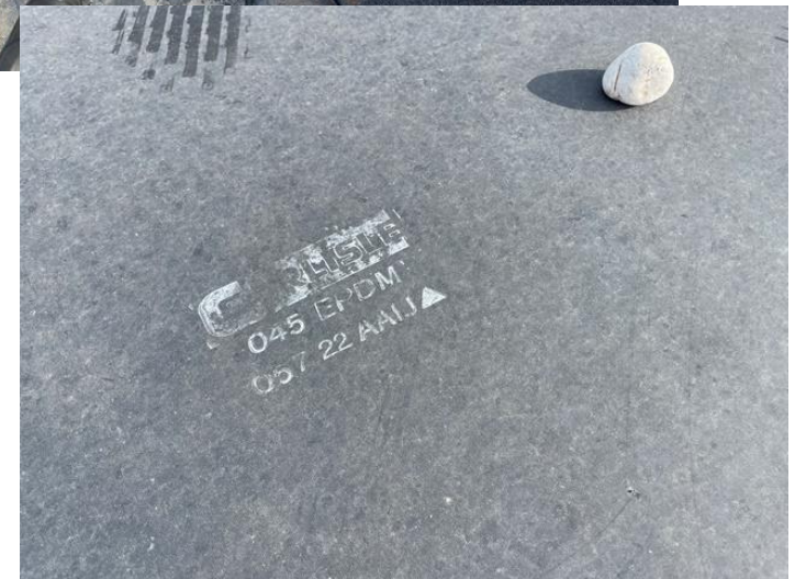
Figure 1 - Existing roof system components include an expanded polystyrene barrier board with ballasted non-reinforced EPDM 45-mil thick membrane. Moisture measured to be high at this location that was an area of existing mechanical damage that had breached the membrane prior to NMBEA's inspection. This location was patched and repaired after testing to prevent further moisture damage.
