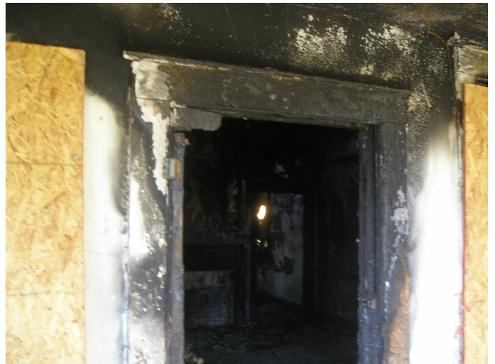
Photo 12 – Front door fire damage.
