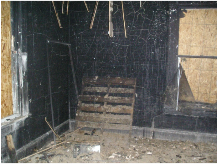
Photo 7 – Typical view of fire damage.
