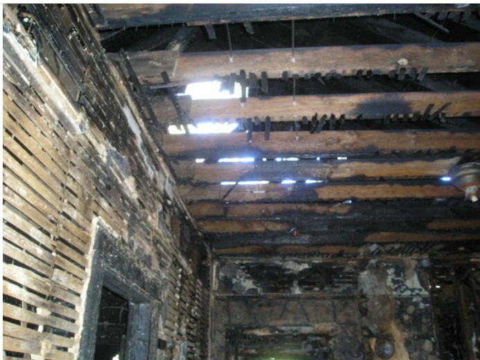
Photo 5 – Typical view of fire damage.
