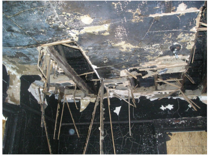
Photo 8 – Typical view of fire damage.
