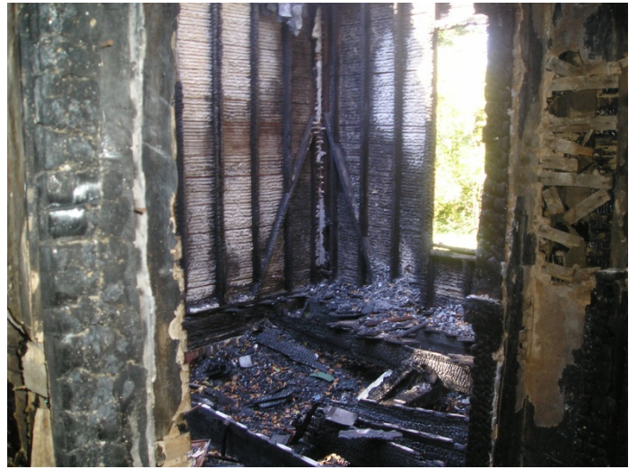
Photo 10 – Typical view of fire damage.
