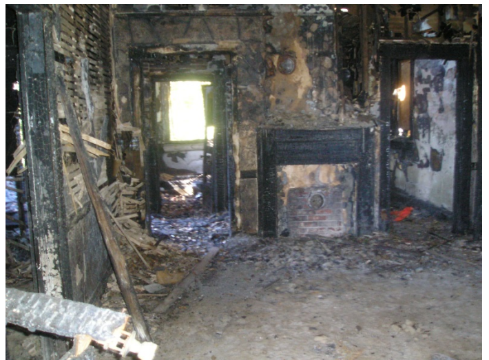
Photo 4 – Typical view of fire damage
