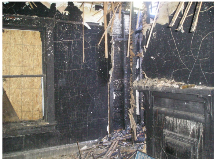
Photo 6 – Typical view of fire damage.
