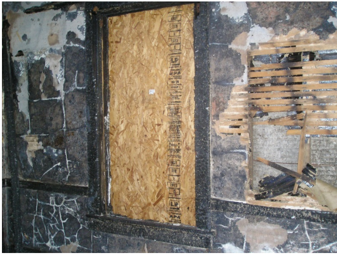
Photo 9 – Typical view of fire damage.
