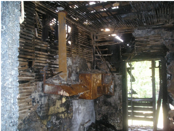
Photo 11 – Kitchen fire damage.
