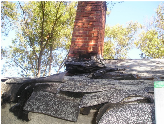
Photo 3 – Chimney with tar.
