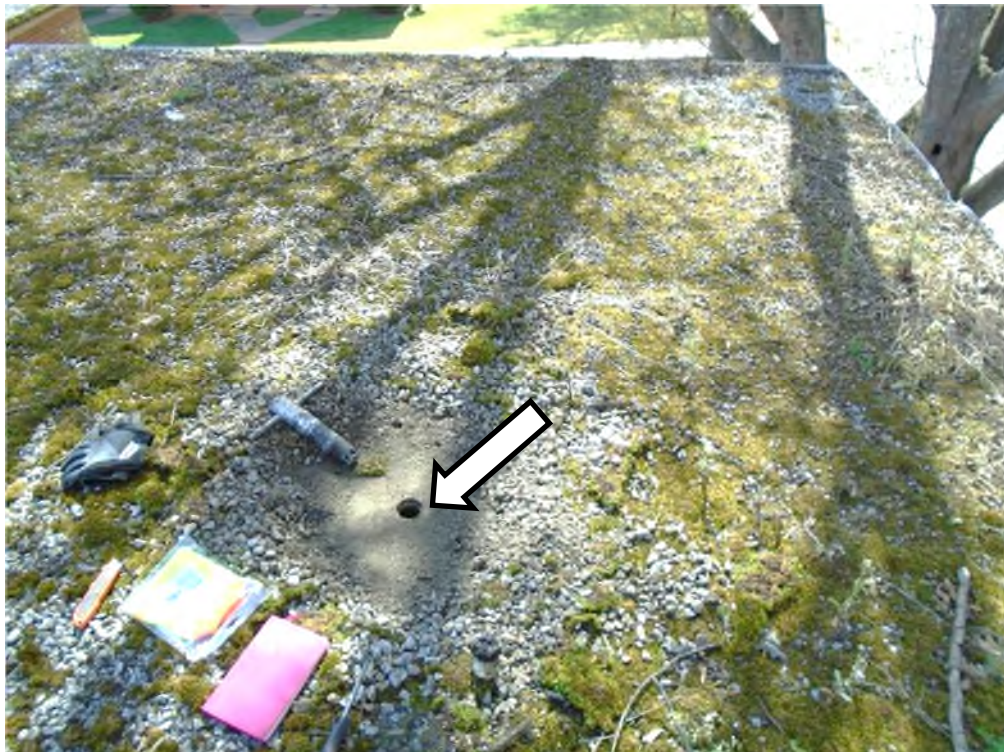
Photograph 20 - BLDG 5 – Wet insulation at core location
