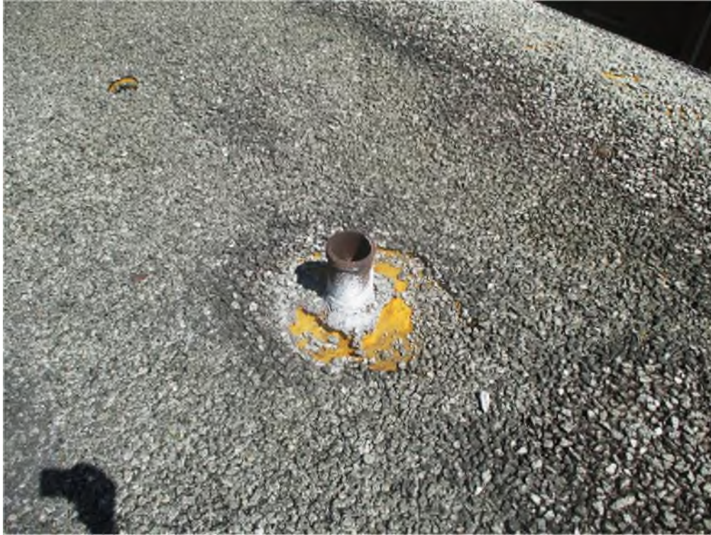
Photograph 31 - BLDG 8 – Deteriorated foam at pipe penetration
