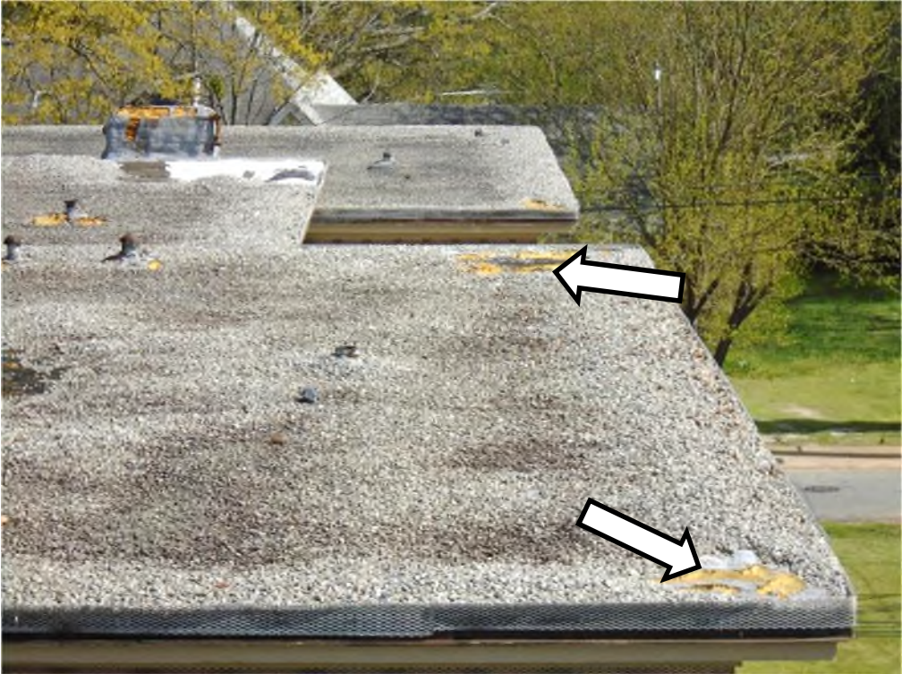
Photograph 42 - BLDG 12 – Deteriorated foam at roof corners
