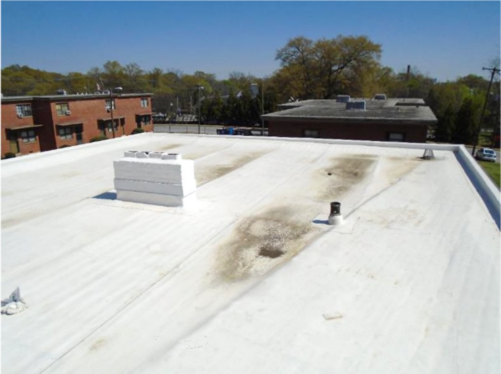
Photograph 21 - BLDG 5 – Minor staining on TPO roof
