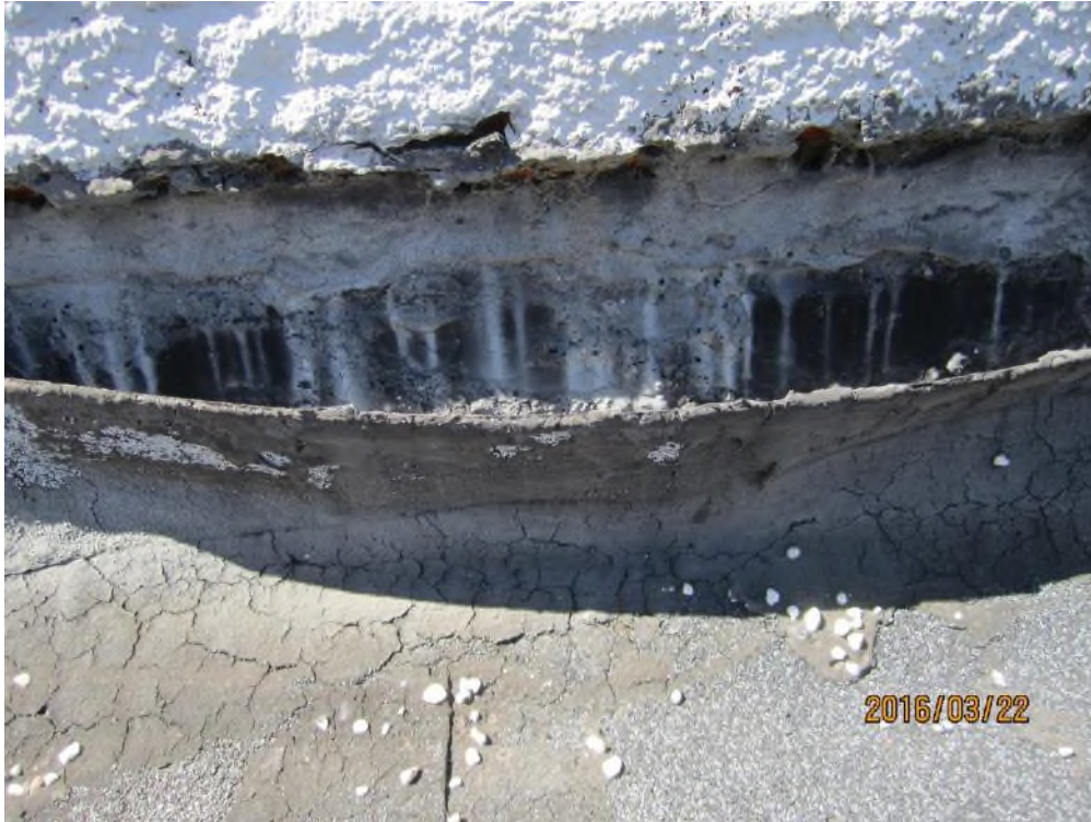
Photograph 37 - BLDG 11 – Loose base flashing at chimney
