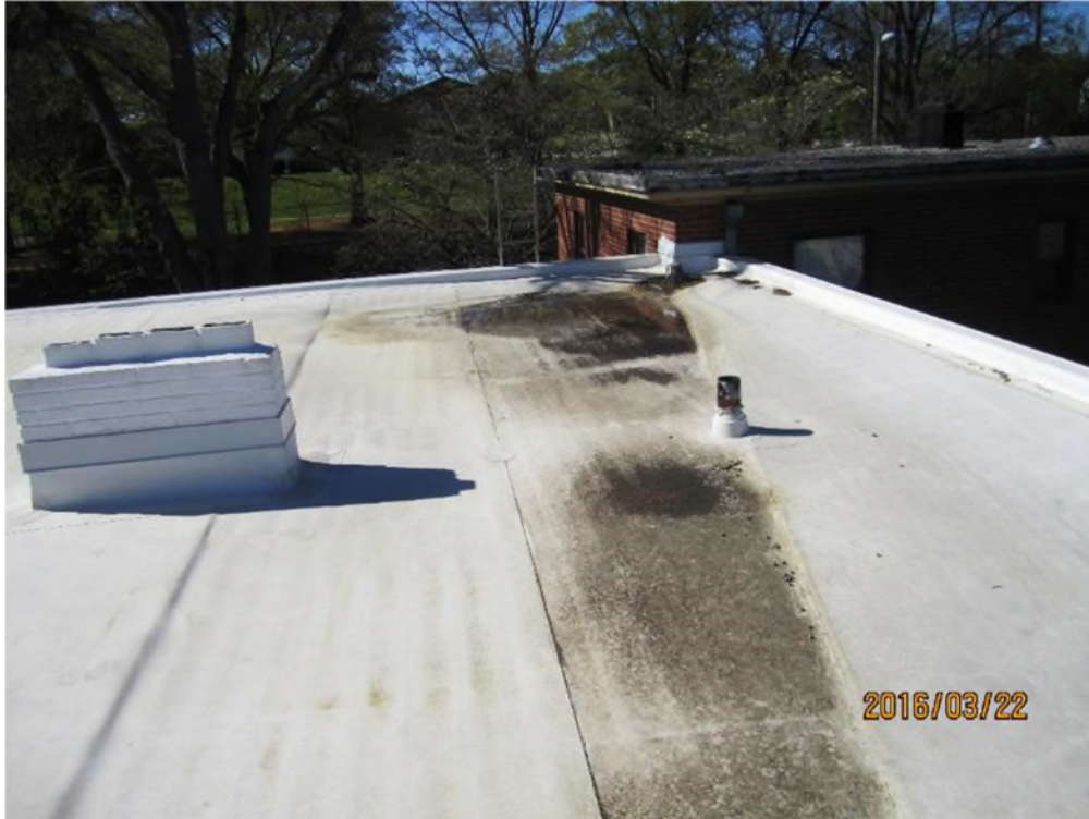
Photograph 25 - BLDG 7 – Minor staining on TPO roof
