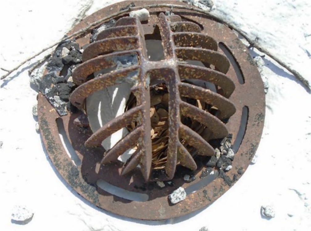
Photograph 18 - BLDG 5 - Damaged strainer and clogged drain
