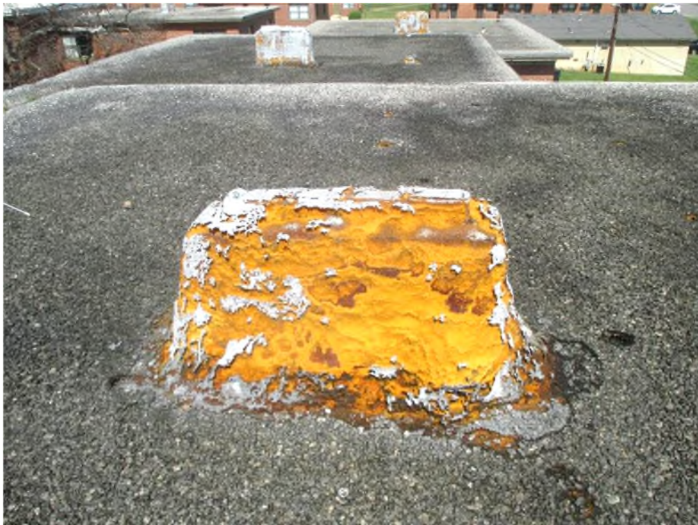
Photograph 32 - Deteriorated foam at chimney
