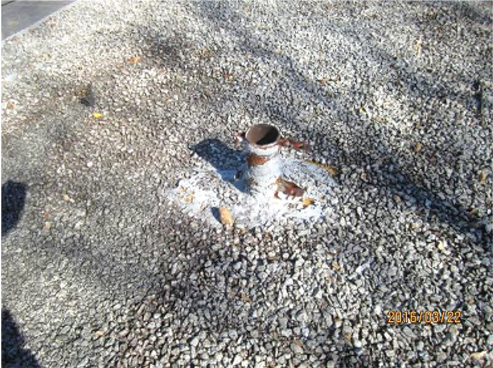
Photograph 27 - BLDG 7 – Deteriorated pipe flashing
