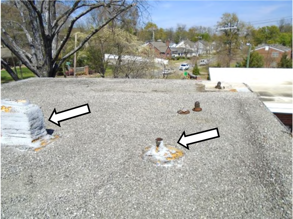
Photograph 12 - BLDG 2 – Deteriorated foam
