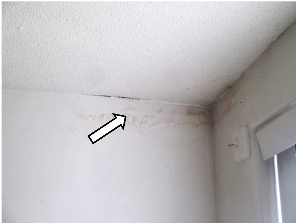
Photograph 8 - BLDG 1 - Moisture staining on ceiling
