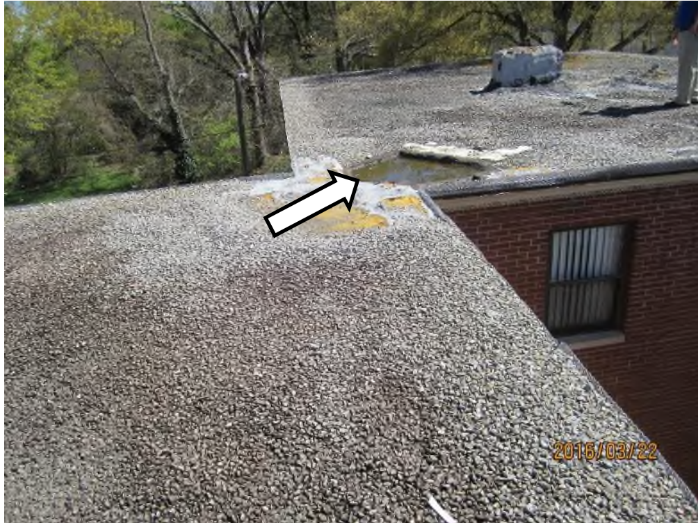
Photograph 39 - BLDG 11 – Water ponded by improper scupper construction
