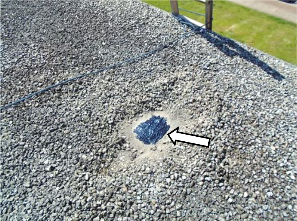
Photograph 11 - BLDG 2 – Wet insulation in test core
