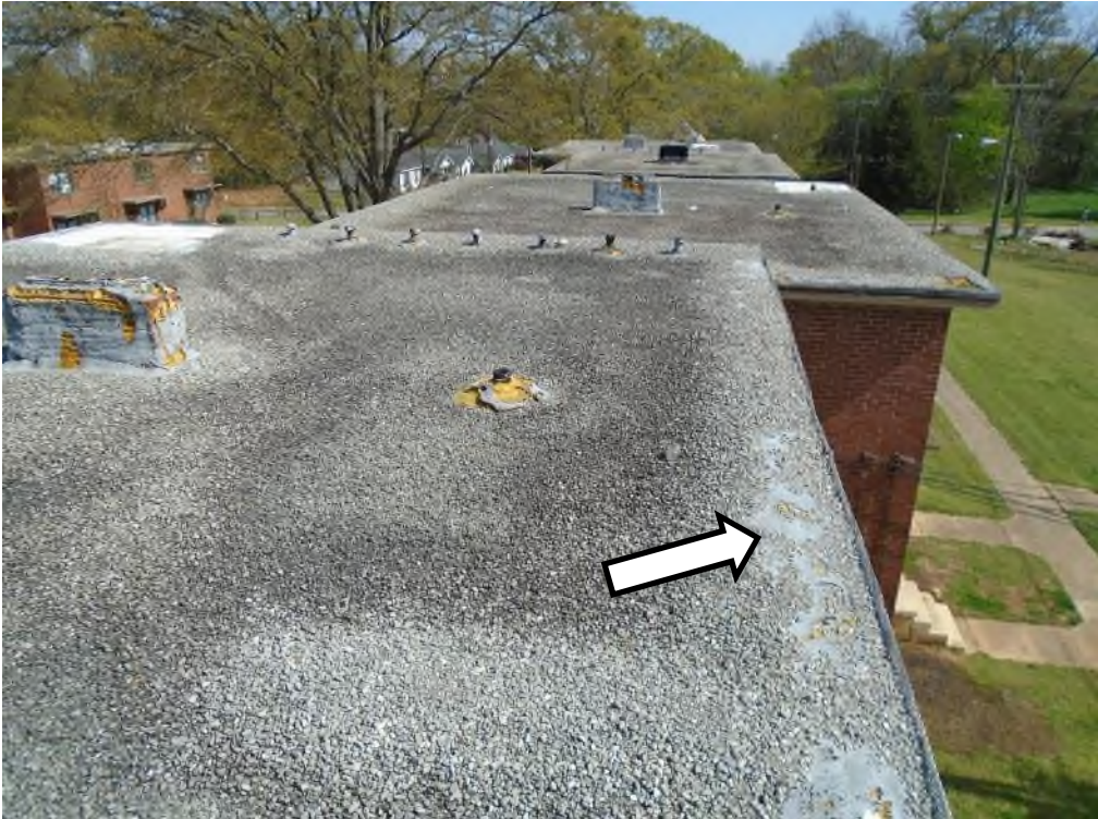
Photograph 45 - BLDG 13 – Deteriorated foam along roof edge
