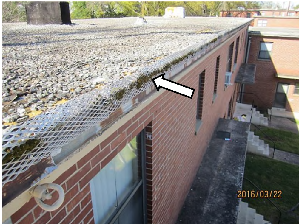
Photograph 26 - BLDG 7 - Vegetation along roof edge
