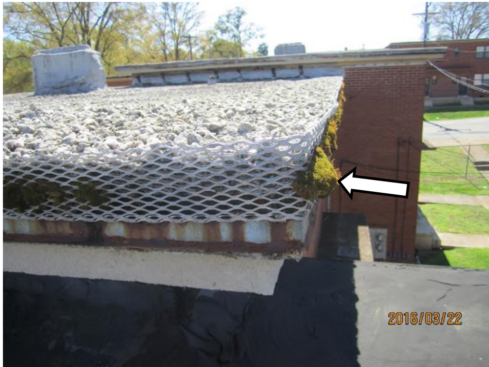
Photograph 38 - BLDG 11 – Vegetation along roof edge
