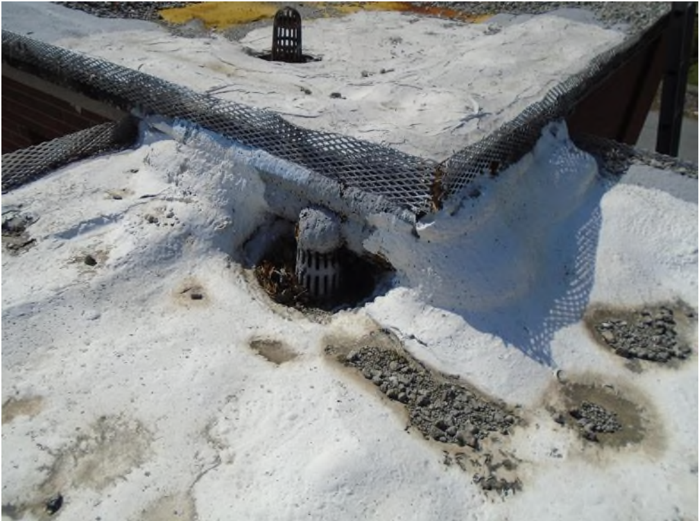
Photograph 46 - BLDG 13 – Multiple repairs to roof at drain
