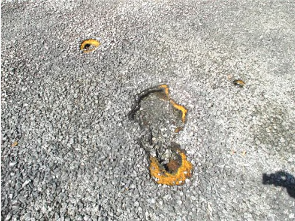
Photograph 30 - BLDG 8 – Voids in roof surface
