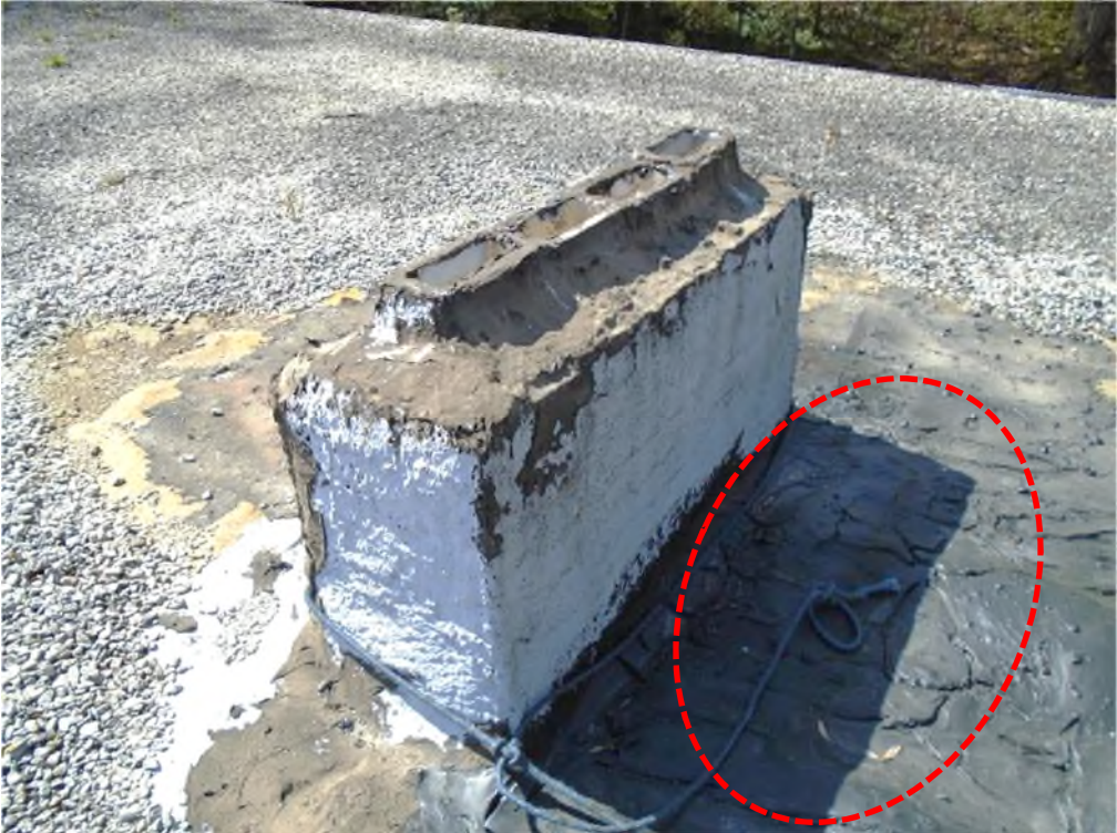
Photograph 17 - BLDG 5 - Failed repair to chimney
