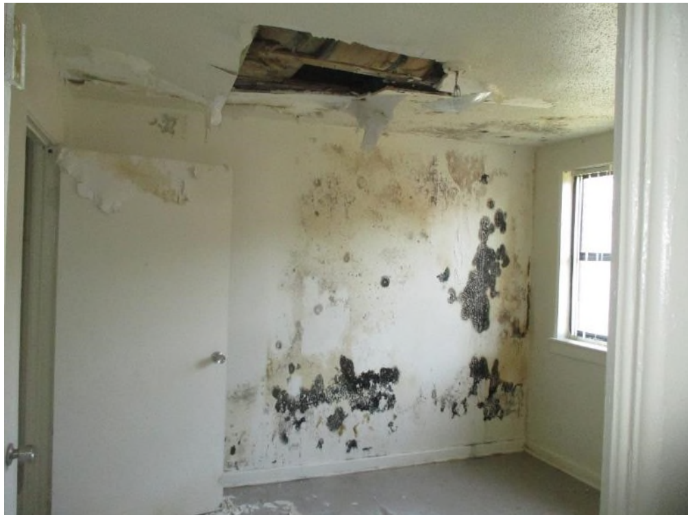
Photograph 40 - BLDG 11 – Partial ceiling collapse and microbial growth
