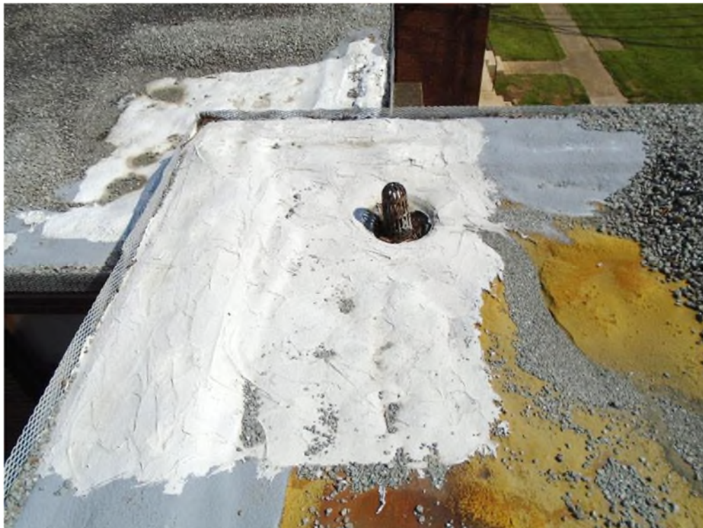
Photograph 44 - BLDG 13 – Multiple repairs made to roof at drain
