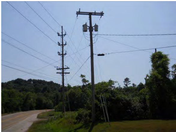
Photo #9 View of a pole mounted electrical transformer located at the site along Hamm Road.
