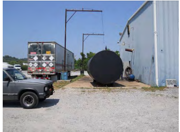
Photo #8 View of the active water AST located at 159 Hamm Road.
