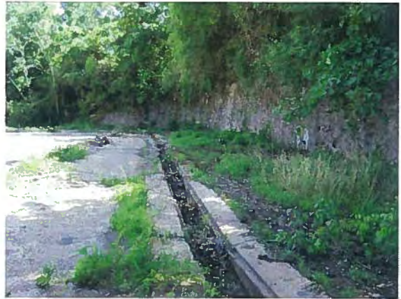
Photo #14 View of the retaining wall and channel drain located at the W. boundary of 155 Hamm Rd.
