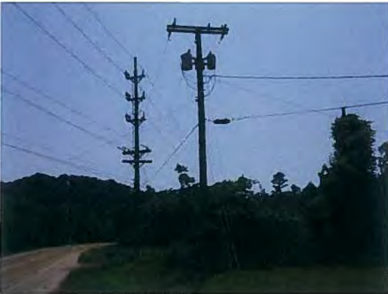
Photo #9 View of a pole mounted electrical transformer located at the site along Hamm Road.
