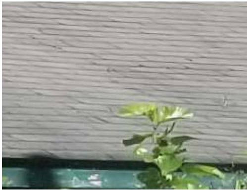
HOMOGENEOUS AREAS 01, 02 ROOF SHINGLE W/FELT PAPER
