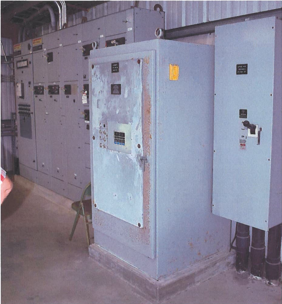
Photo 11 (1,000 Automatic Transfer Switch on 4" raised housekeeping pad)
