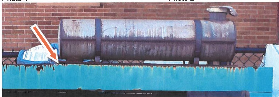
Photo 3 Muffler flange rusted and warped exposing interior to rain
