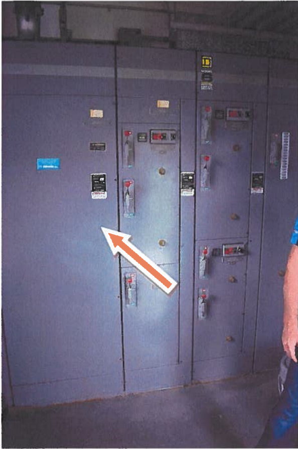
Photo 9 (Motor Control Center, ATS cabinet (orange))
