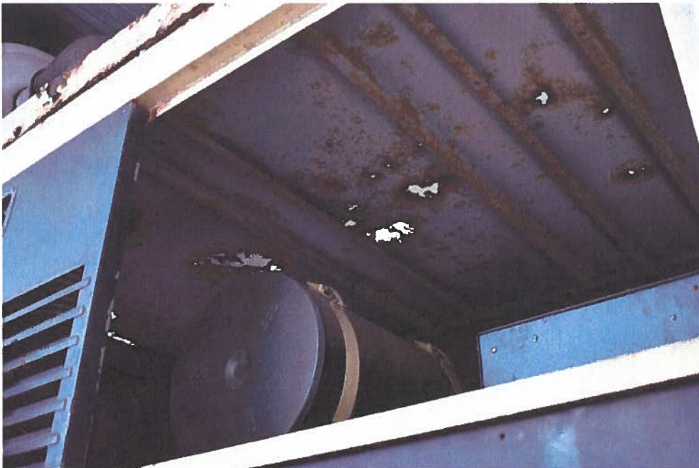
Photo 9 (this is the rusted out roof of the generator enclosure)
