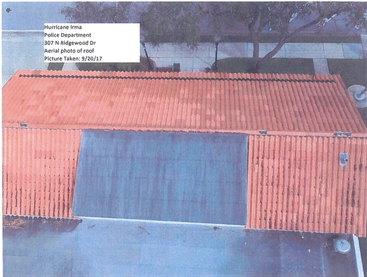
View of Hurricane Irma roof damage and failing internal roof gutter system
