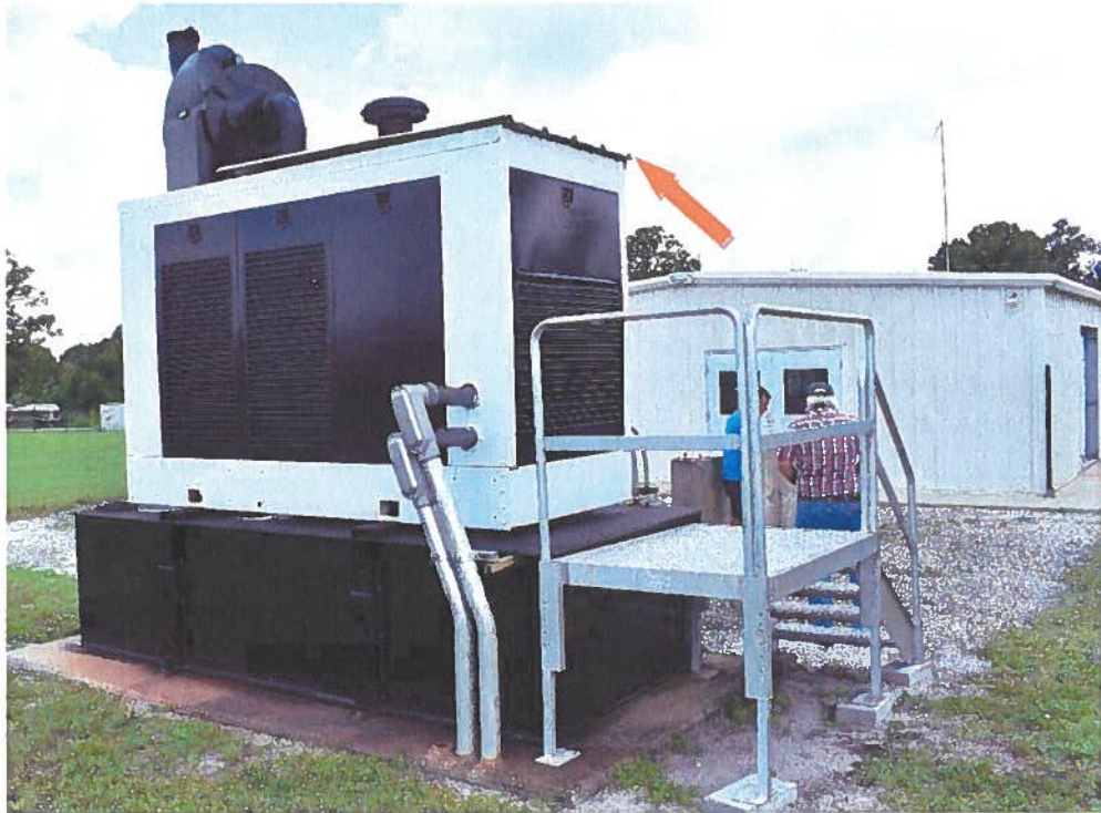
Photo 5 (corrugated metal screwed to top of generator enclosure)
