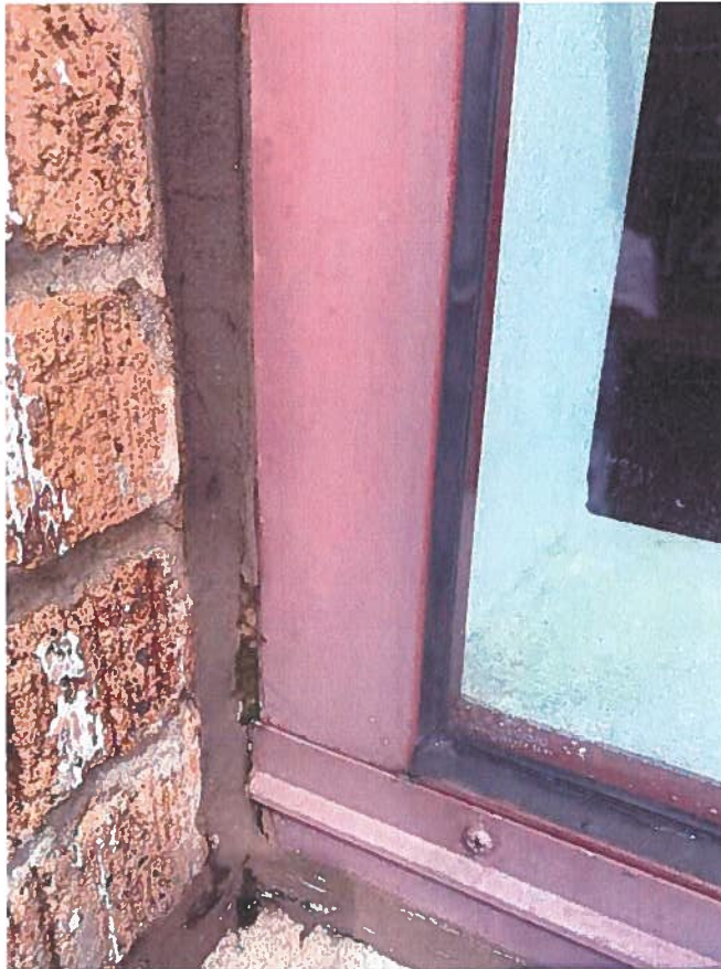
View of existing steel impact windows that only meet Large Missile D testing requirements, not Large Missile E testing requirements
