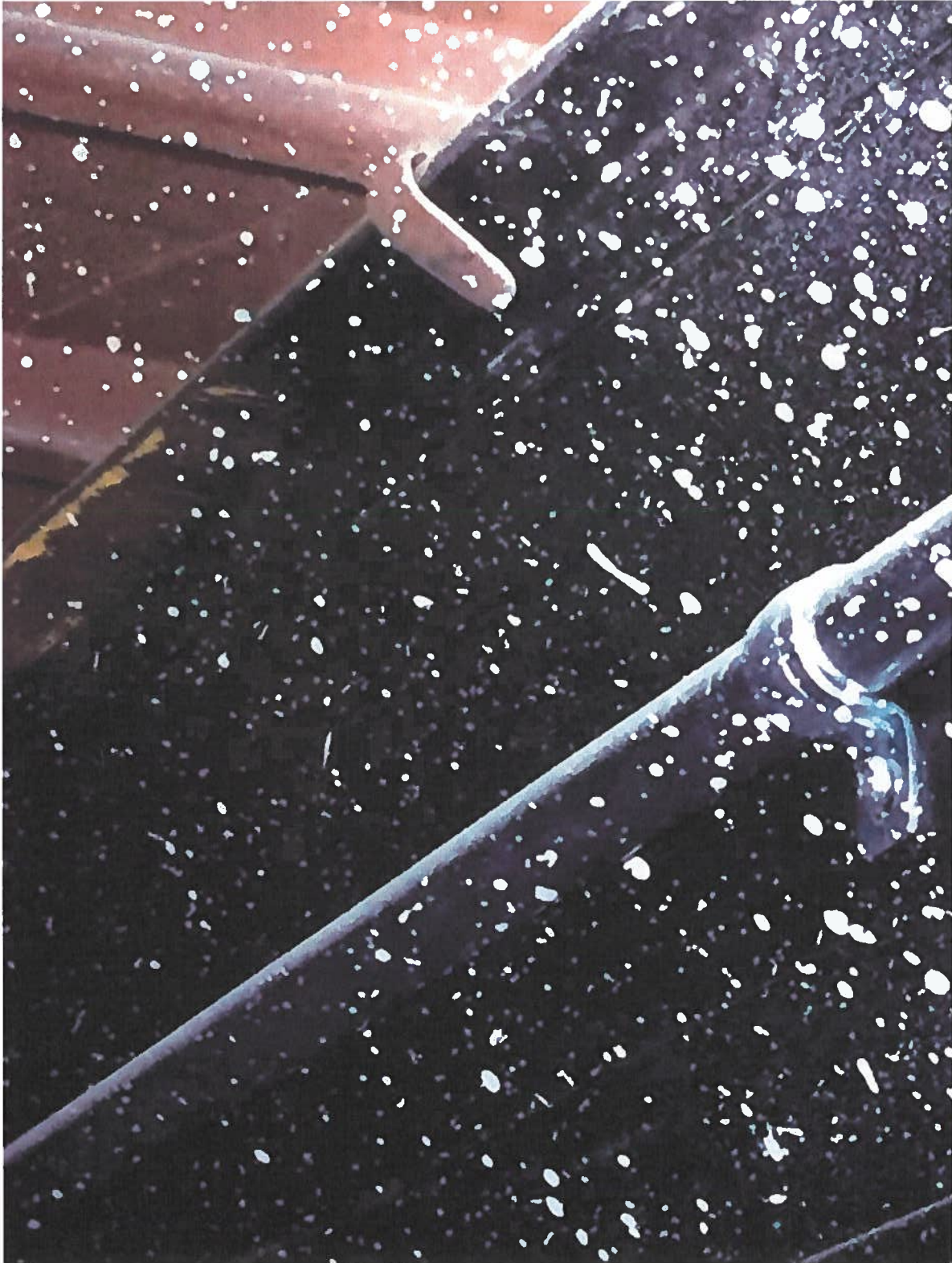
Photo 5: Existing Metal Roof Deck Hold-Down Bent Tab
