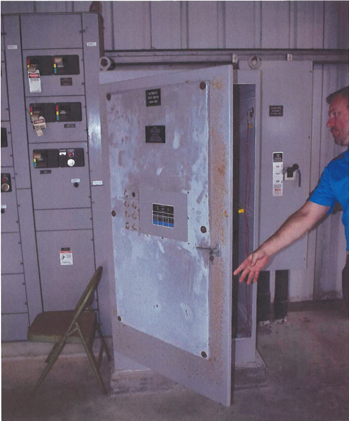
Photo 8 (Existing 1,000 Ampere Transfer Switch in custom cabinet)
