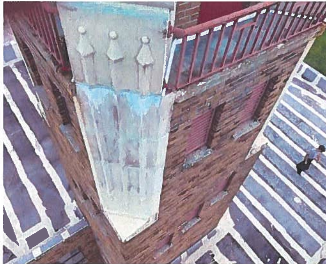
View of loose brick mortar that needs to be tuck pointed and degraded vent and window limestone sills that need to be replaced
