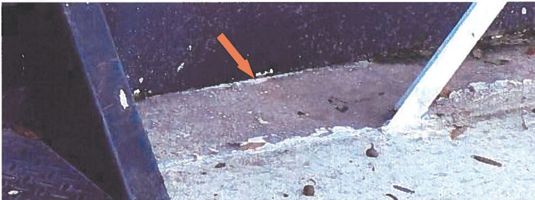
Photo 11 (close up of photo 10, steel fuel tank resting on concrete without air space)
