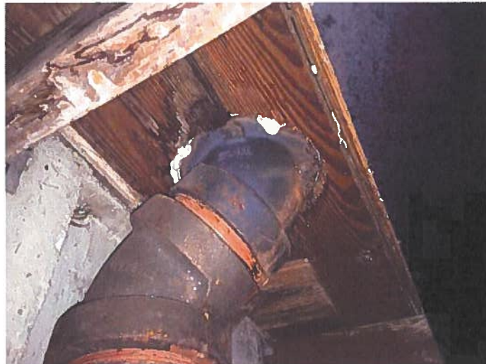
View of the internal roof gutter with evidence of water intrusion
