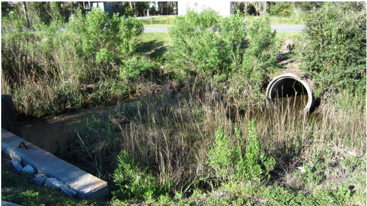
Duck Pond outlet pipe (left); Battery Creek Road 24-inch crossline pipes (right)
