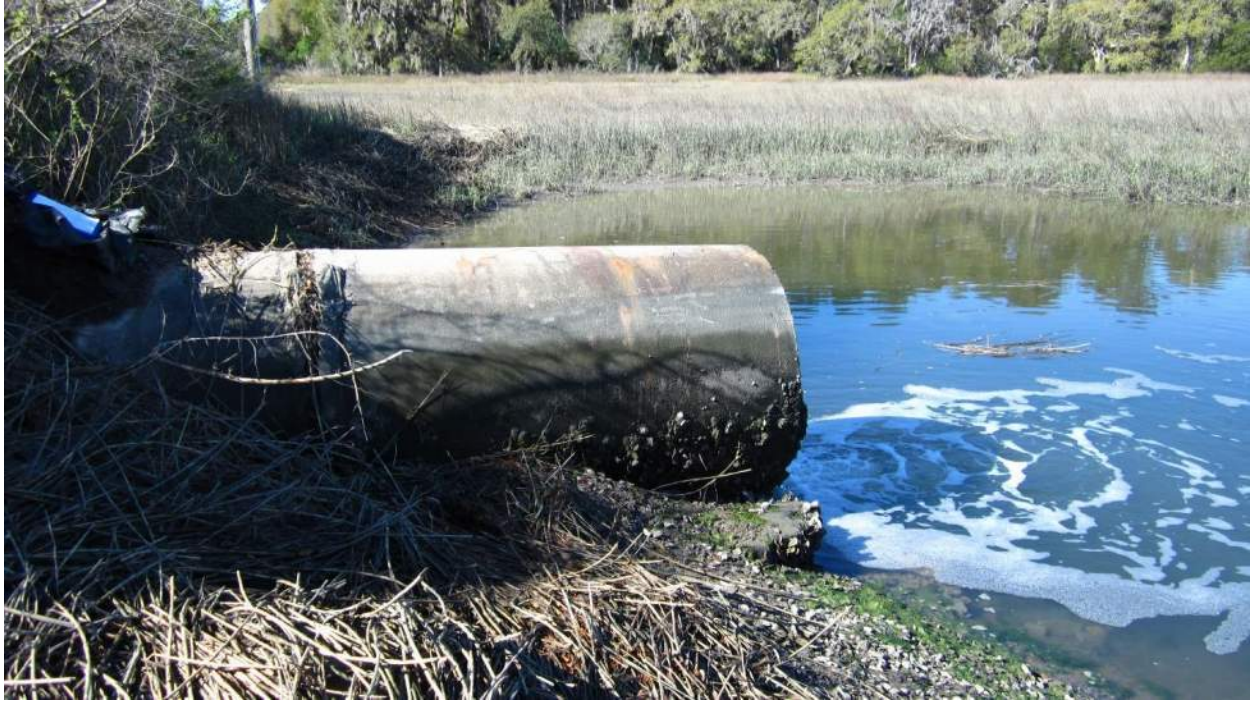
Outlet end of Spanish Moss Trail 48-in crossline pipe
