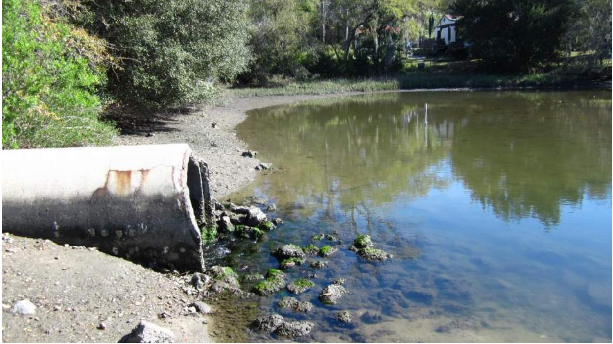
Upstream (Mossy Oaks) end of Spanish Moss Trail 48-in crossline pipe
