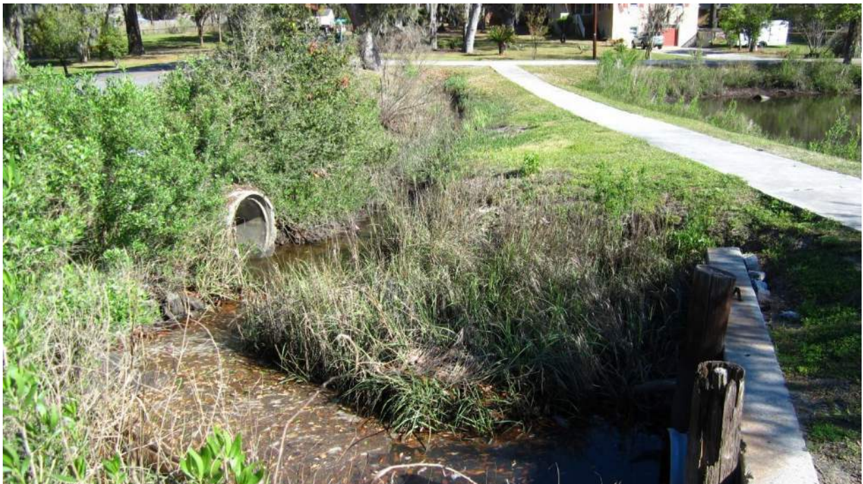
Battery Creek Road 24-inch crossline pipes (left); Duck Pond 36-inch CMP outlet pipe (right)
