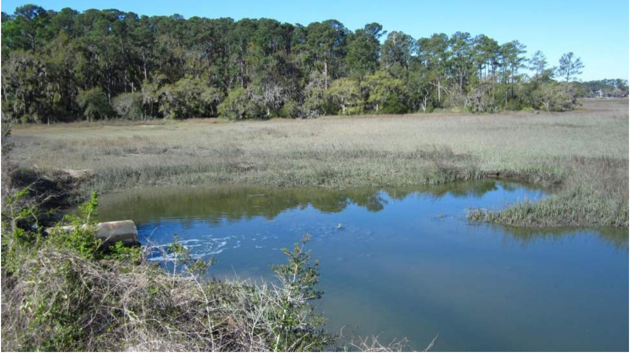
Downstream (Battery Creek) end of Spanish Moss Trail 48-in crossline pipe
