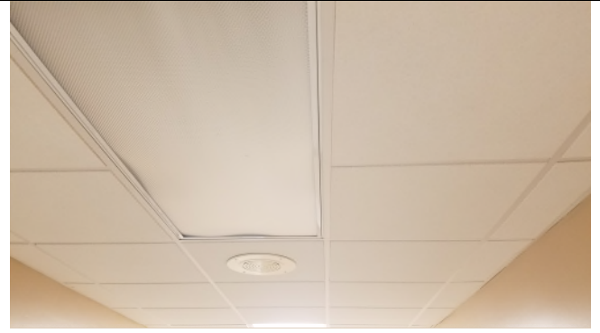
Picture 14 – *HA30 2x2 Textured Ceiling Tiles
