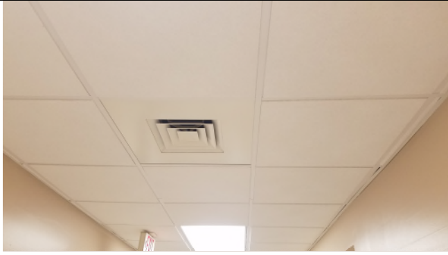
Picture 13 – *HA30 2x2 Textured Ceiling Tiles
