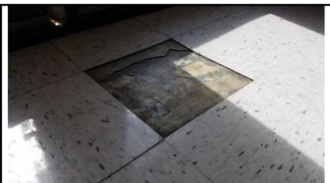
Picture 6 – White 12x12 Floor Tiles w/Mastic (Not Included in Scope of Renovation)
