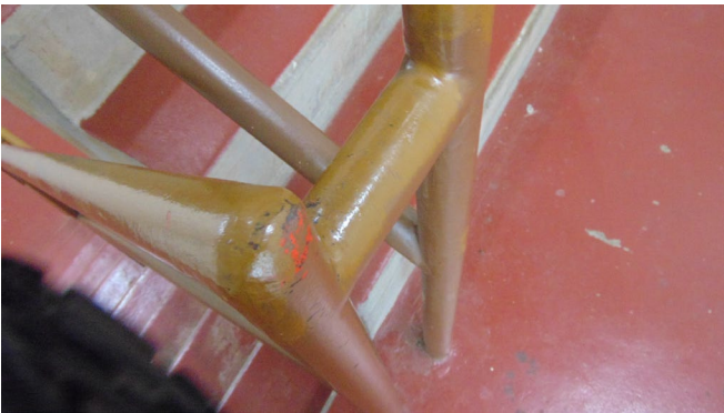
Stairwell Handrail – Deteriorated LBP
