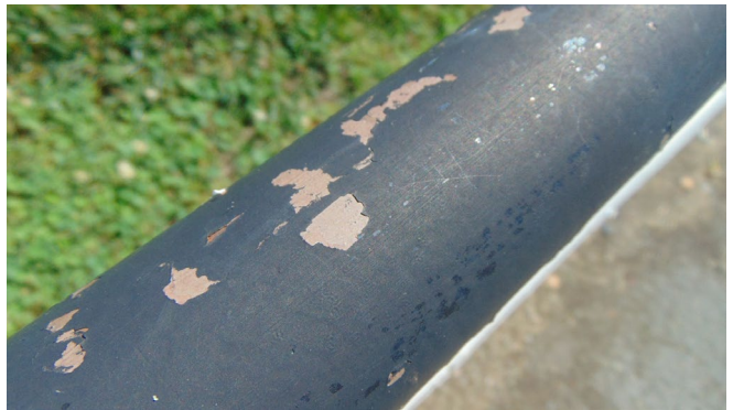
Exterior Handrail – Deteriorated LBP
