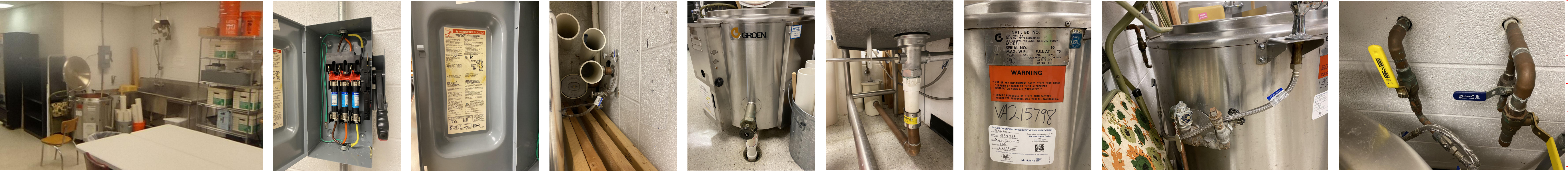
EXISTING PHOTOS OF R-58 STEEL SINK AND DYE VAT AT GUNSTON MS
