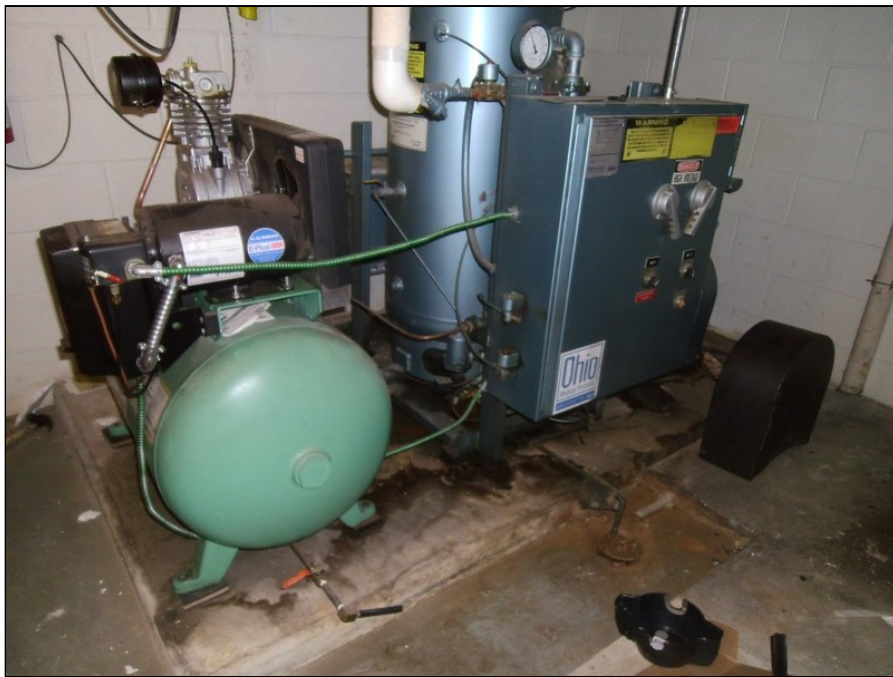
12 - View of basement boiler mechanical room.
