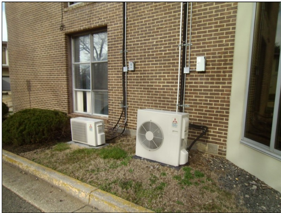
18 - View of typical room unit HVAC equipment.
