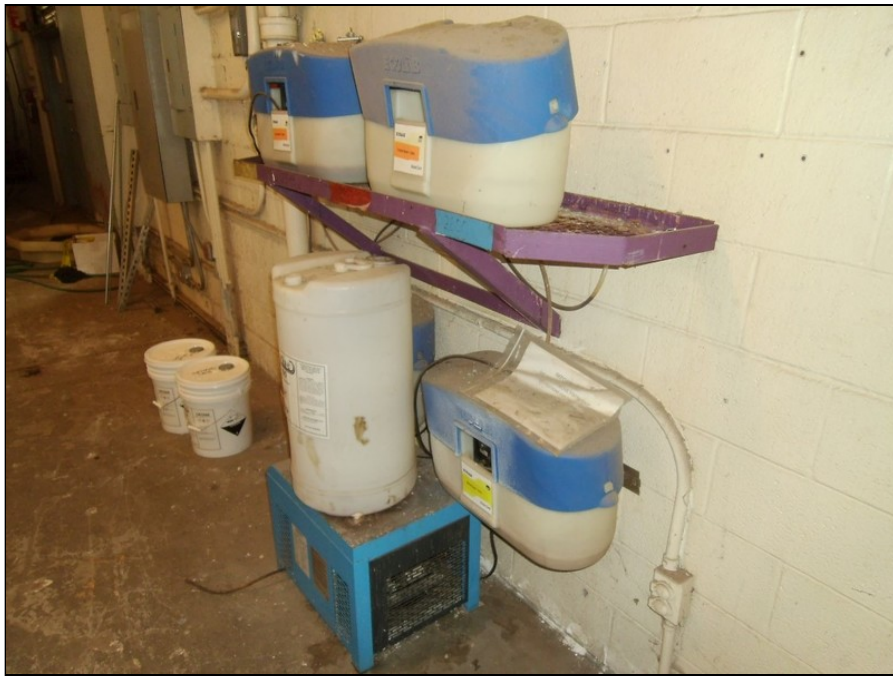
15 - View of water treatment equipment within basement mechanical room.
