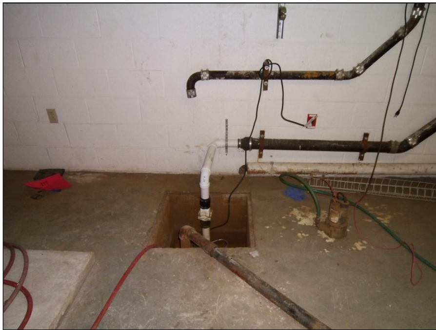
14 - View of typical sump pit within basement mechanical room.
