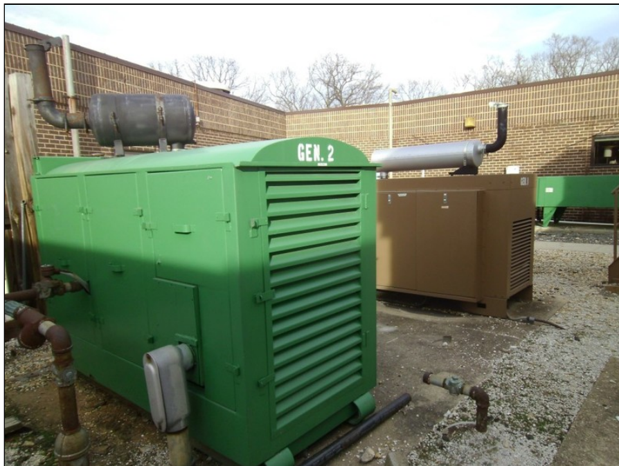
8 - View of Generator 1 & 2.
