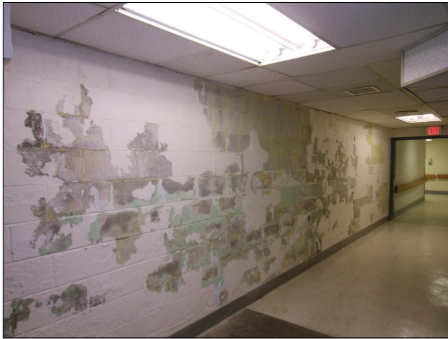
17 - View of water damage to basement masonry walls.
