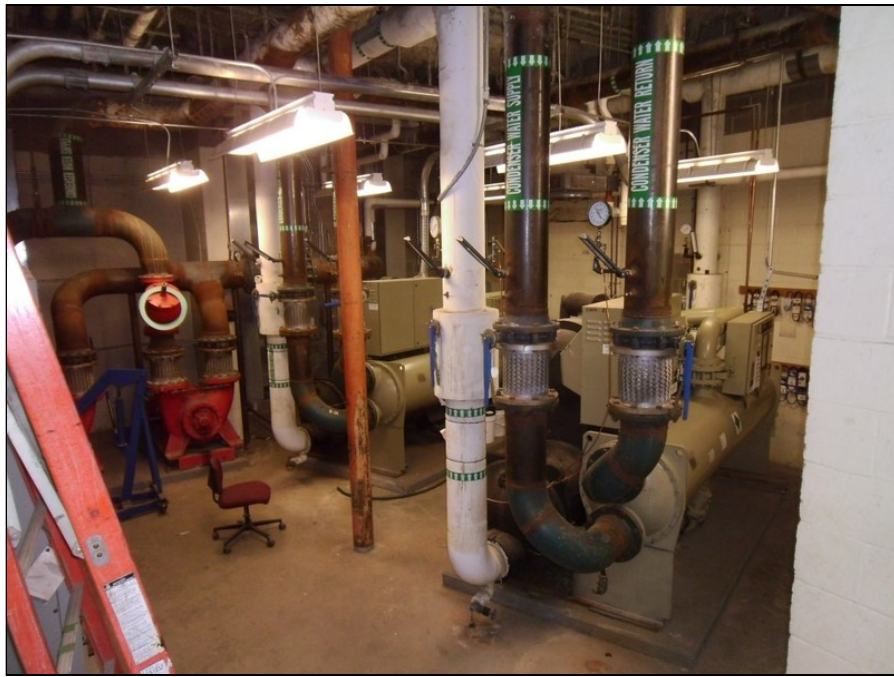
13 - View of basement boiler mechanical room.
