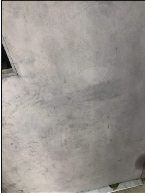
9 - View of Lead Based Paint on a Dark Gray Metal Door. XRF Reading Nos. 1050 and 1051.
