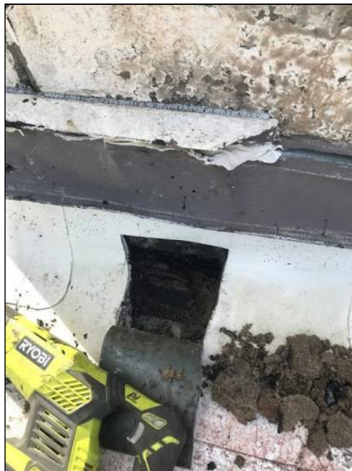
2 - View of Asbestos-Containing Multiple Layered Flashing Caulk on the Connecting Building Parapet Wall. Sample No. 61.
