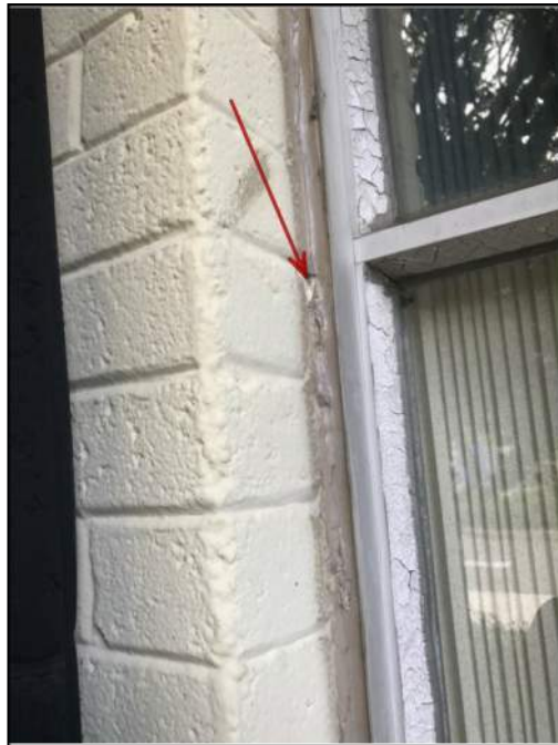
4 - View of Asbestos-Containing White Window Caulk on Exterior Windows. Sample No. 127-B.
