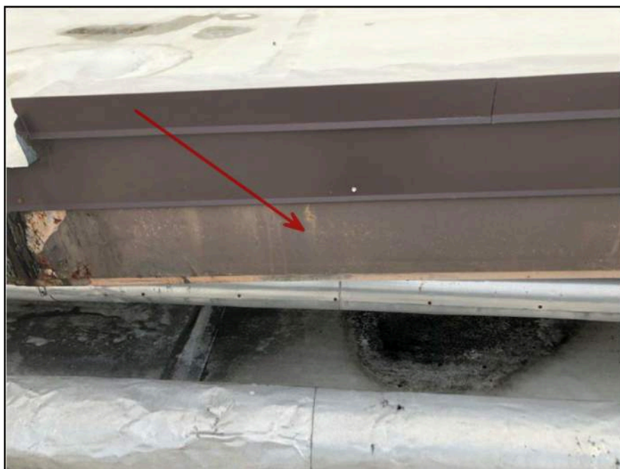
8 - View of Lead Based Paint on a Red Metal Beam on the Roof. XRF Reading No. 1031.
