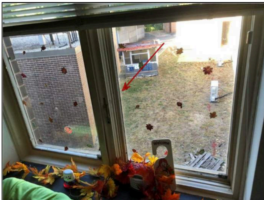
7 - View of Asbestos-Containing Interior Black Window Glazing on Connecting Building Windows. Sample No. 179.
