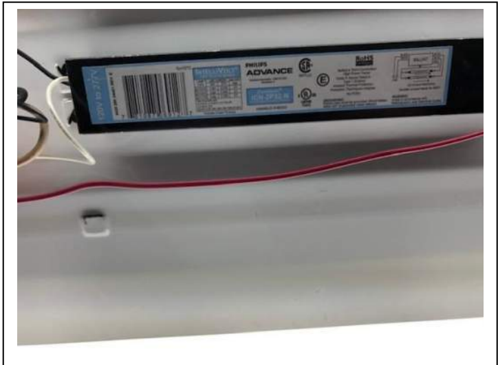
Photo #50 Material: Non-PCB Ballast Sample Result: Not sampled
