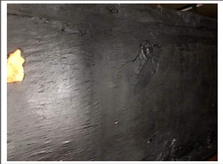
Photo #65 Material: Black Mastic On Canvas Duct Sample Result: 5% Chrysotile
