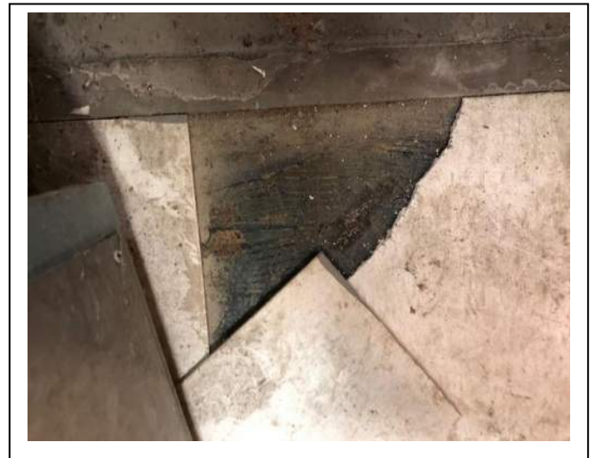
Photo #36 Material: Black Floor Tile Mastic Sample Result: 3-5% Chrysotile
