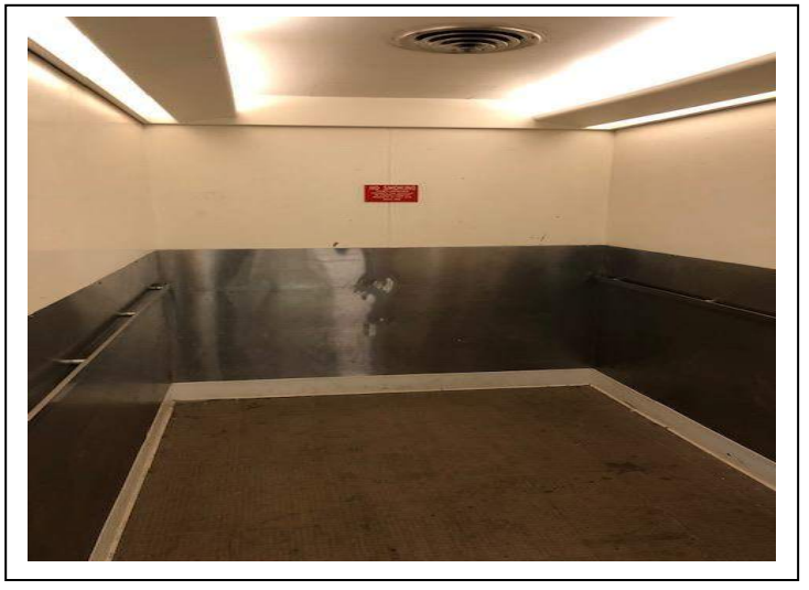
Photo #84 Material: Elevator Cab Insulation Sample Result: Assumed ACM
