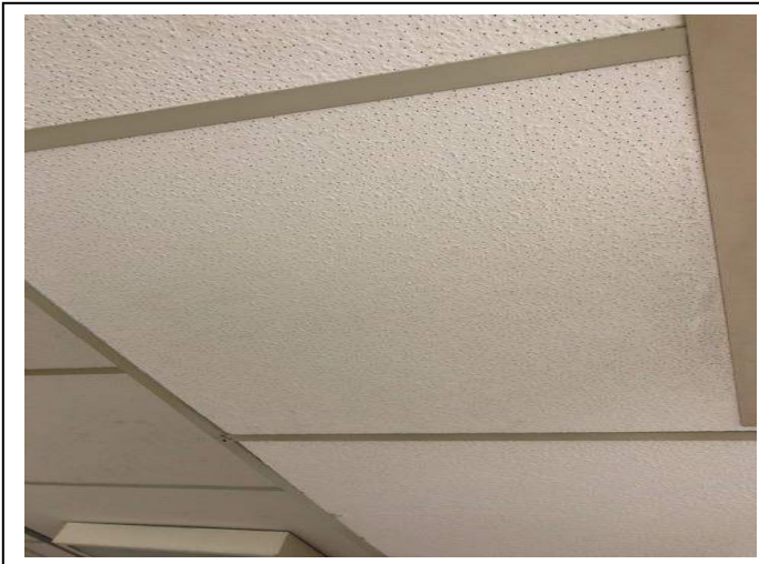
Photo #15 Material: 2'x4' small pinhole ceiling tile Sample Result: No Asbestos Detected
