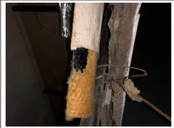
Photo #39 Material: Black Mastic On Fiberglass Insulation Sample Result: 5% Chrysotile
