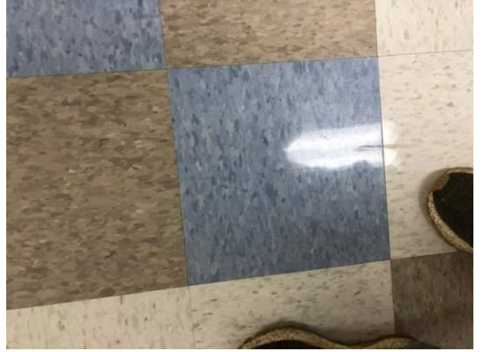
Photo #70 Material: 12"x12" Blue Mottled Floor Tile Sample Result: No Asbestos Detected
