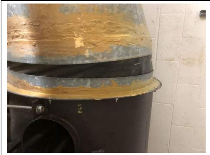
Photo #49 Material: Tan Duct Seam Sealant On Metal Sample Result: No Asbestos Detected
