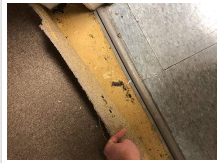
Photo #45 Material: Black Mastic Underneath Yellow Carpet Mastic Sample Result: 2% Chrysotile
