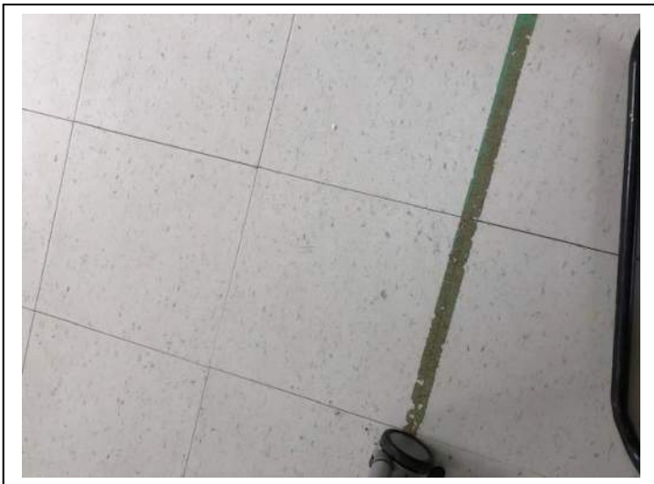
Photo #51 Material: 12"x12" White With Green Specks Floor Tile Sample Result: No Asbestos Detected
