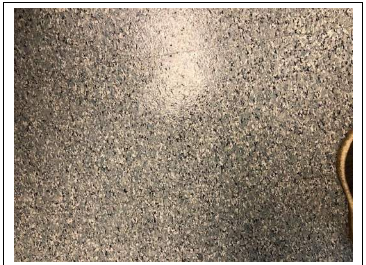
Photo #76 Material: 12"x12" Blue Multi-Speck Floor Tile Sample Result: No Asbestos Detected
