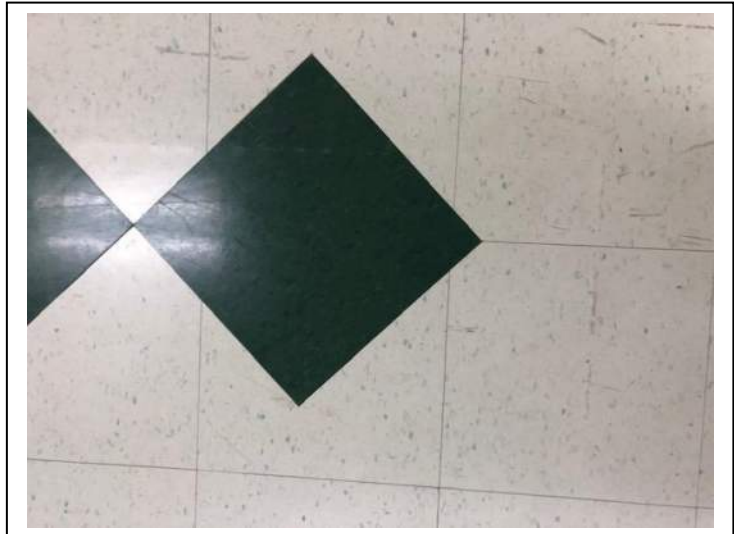
Photo #54 Material: 12"x12" Green Mottled Floor Tile Sample Result: No Asbestos Detected
