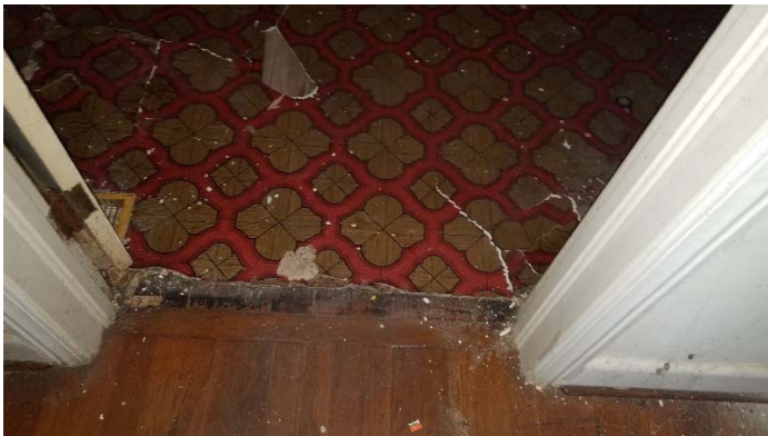
Photo 9 – Front left bedroom flooring.
