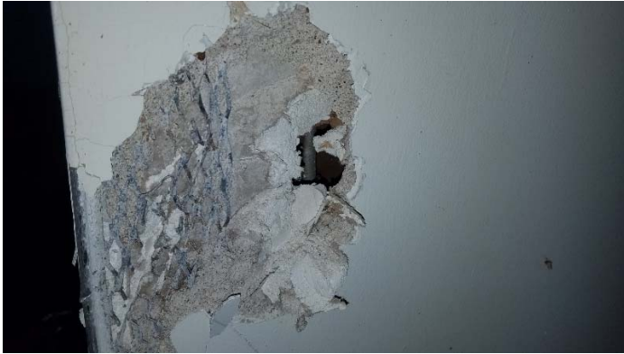
Photo 7 – Plaster over unfinished drywall.
