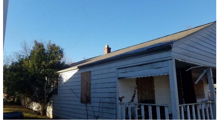
Photo 2 – Assumed asbestos chimney tar.
