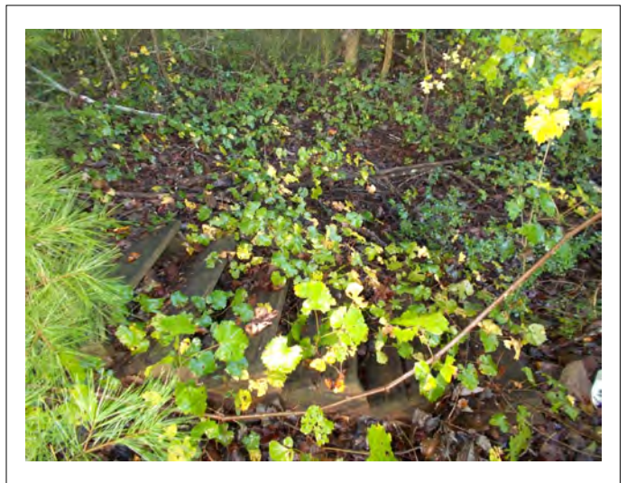
Stairs in the woods along the western boundary of the subject property, facing west.
