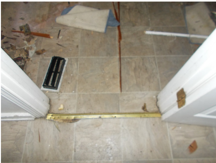
Photo 11 – Tan slate pattern vinyl floor with mastic
