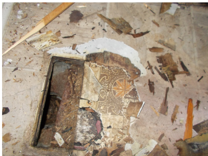
Photo 13 – Multiple layers of vinyl floor with no mastic, floor tile with mastic and felt backing in the kitchen
