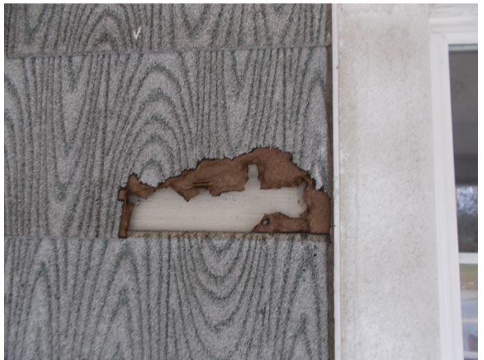
Photo 4 – Composite siding with shingle and felt.
