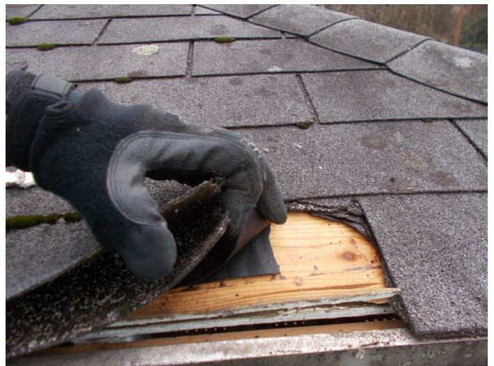
Photo 2 – Roll shingle roof (2) & felt (2).
