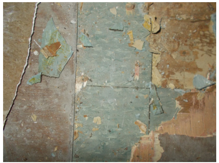
Photo 14 – Green streaked floor tile with mastic over cream vinyl floor with mastic .
