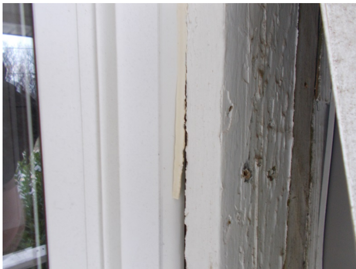
Photo 5 – Window casing caulk.
