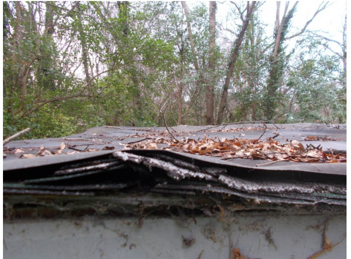
Photo 8 – Roofing shingles (7 layers) and no felt on shed roof.
