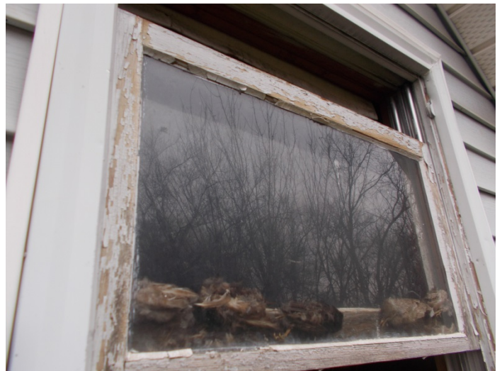
Photo 4 – Wooden window glazing.
