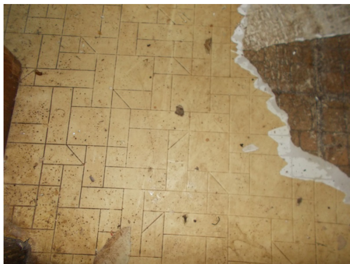
Photo 17 – Cream rectangle pattern vinyl floor with mastic in mud porch (top layer).
