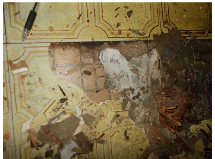
Photo 18 – Brown small square pattern vinyl floor with mastic in kitchen and mud porch (bottom layer).
