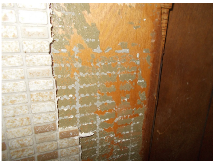
Photo 11 – Wall panel mastic in front right bathroom.
