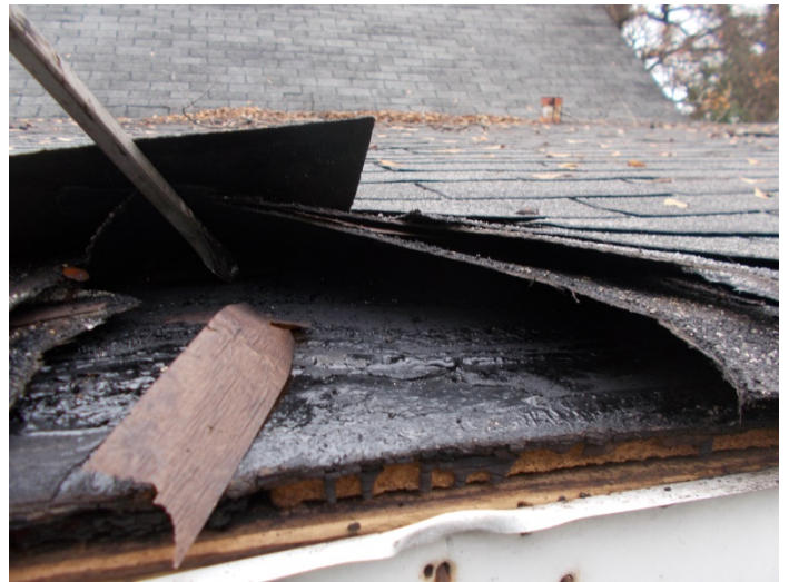
Photo 2 – Roof shingles (2 layers) with tar and no felt.
