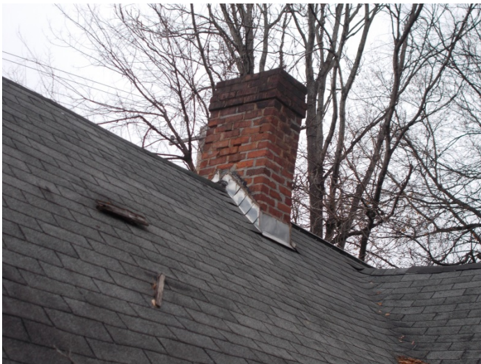
Photo 3 – One chimney with tar assumed positive.
