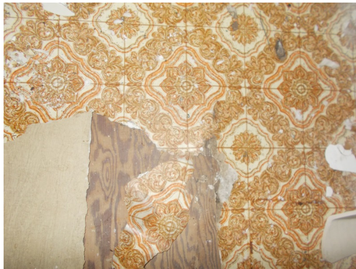
Photo 15 – Brown and orange pattern vinyl floor with mastic in rear bathroom.
