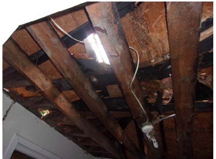
Photo 12 – View of collapsed roof and ceiling
