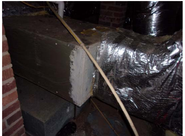
Photo 4 – Beige HVAC mastic in crawlspace & on HVAC
