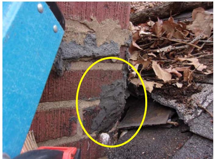
Photo 6 – Tar on 2 chimneys
