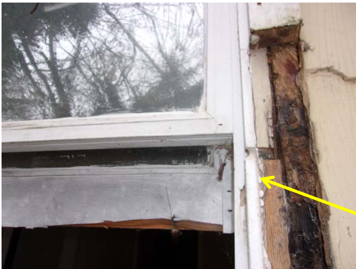
Photo 5 – Bid wooden windows with caulk
