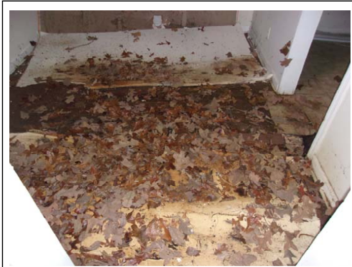
Photo 13 – View of unstable flooring
