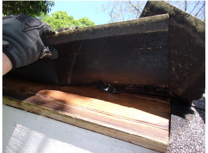
Photo 2 – Roof shingles with tar and no felt
