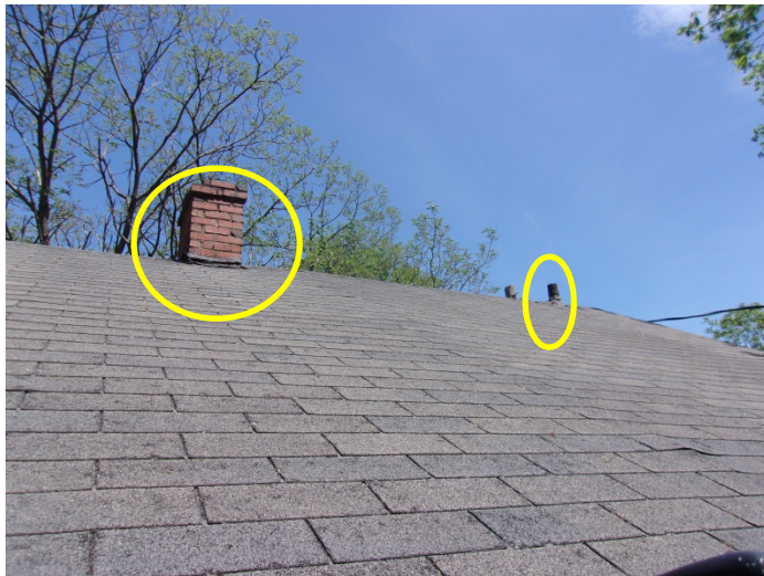
Photo 3 – Tar on chimney & vent pipe – assumed positive
