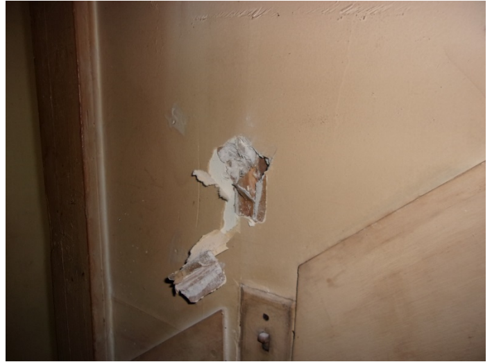
Photo 8 – Drywall with joint compound & tape in the back right bedroom walls & ceiling
