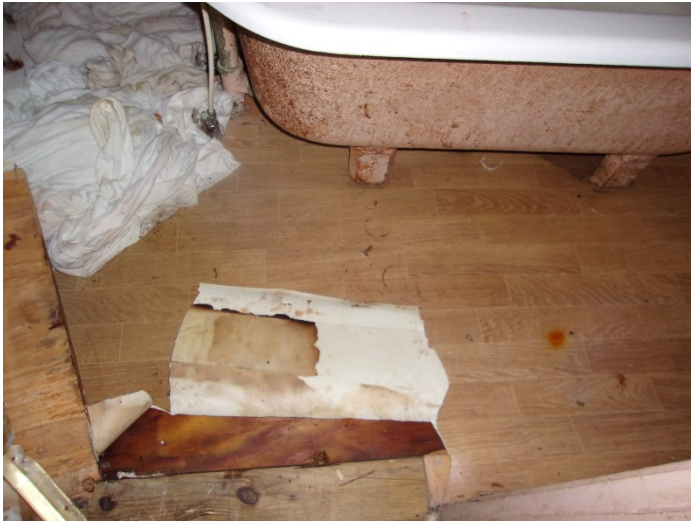
Photo 9 – Brown wooden plank pattern vinyl floor with no mastic in the bathroom
