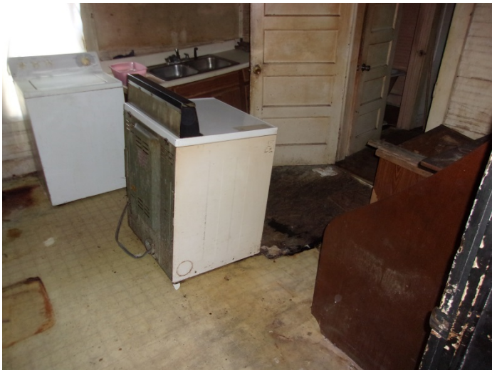
Photo 11 – The flooring is unstable and collapsed in some areas of the kitchen
