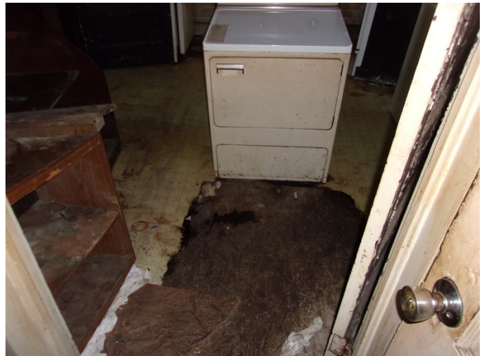
Photo 12 – The flooring is unstable and collapsed in some areas of the kitchen
