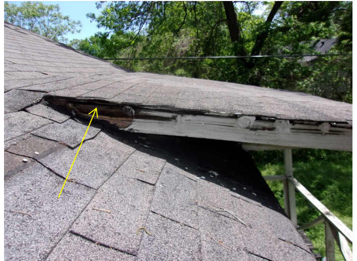
Photo 4 – Tar on roof line at the side porch – assumed positive
