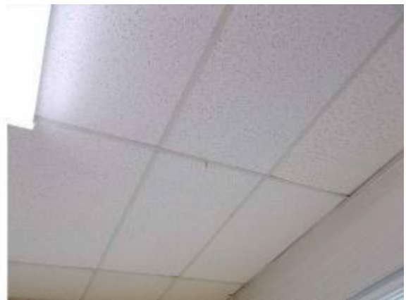
Photo #12 View of the drop ceiling tile in the original main building.
