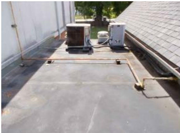
Photo #9 View of the roof of the breezeway. Flashing material identified as asbestos containing.
