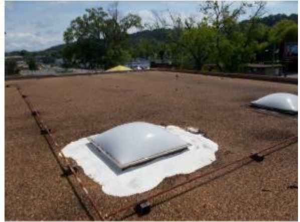
Photo #8 View of the roof of the gymnasium building. Flashing material identified as asbestos containing.
