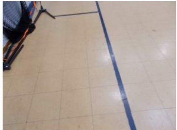
Photo #22 View of the asbestos containing floor tile (HA-30) in the gymnasium.
