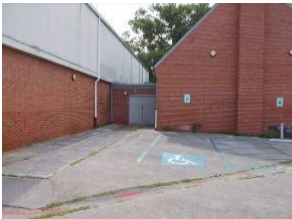
Photo #5 View of the exterior of the breezeway between the original main building and the gymnasium.
