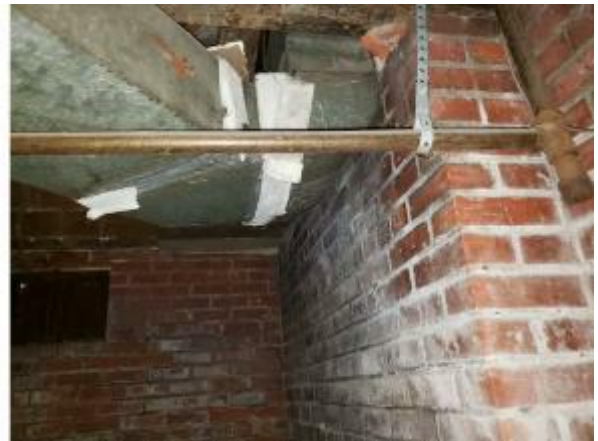
Photo #24 View of the asbestos containing tape (HA-34 and HA-35) on the duct work in the basement.
