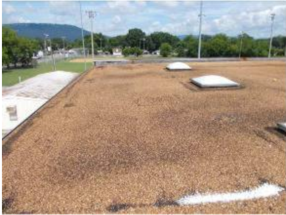
Photo #7 View of the roof of the gymnasium building. Note: Flashing material identified as asbestos containing.
