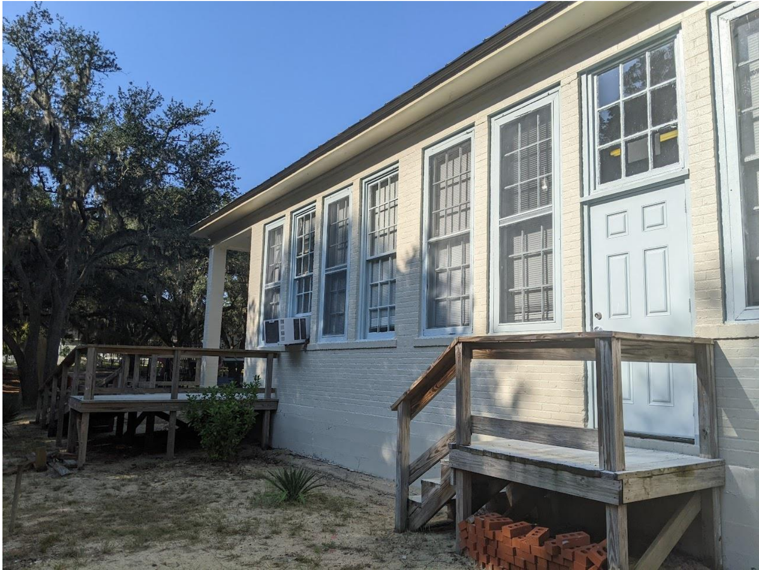
Exterior steps & ramp to be demoed to create new ADA ramp that connects to front & back door.
