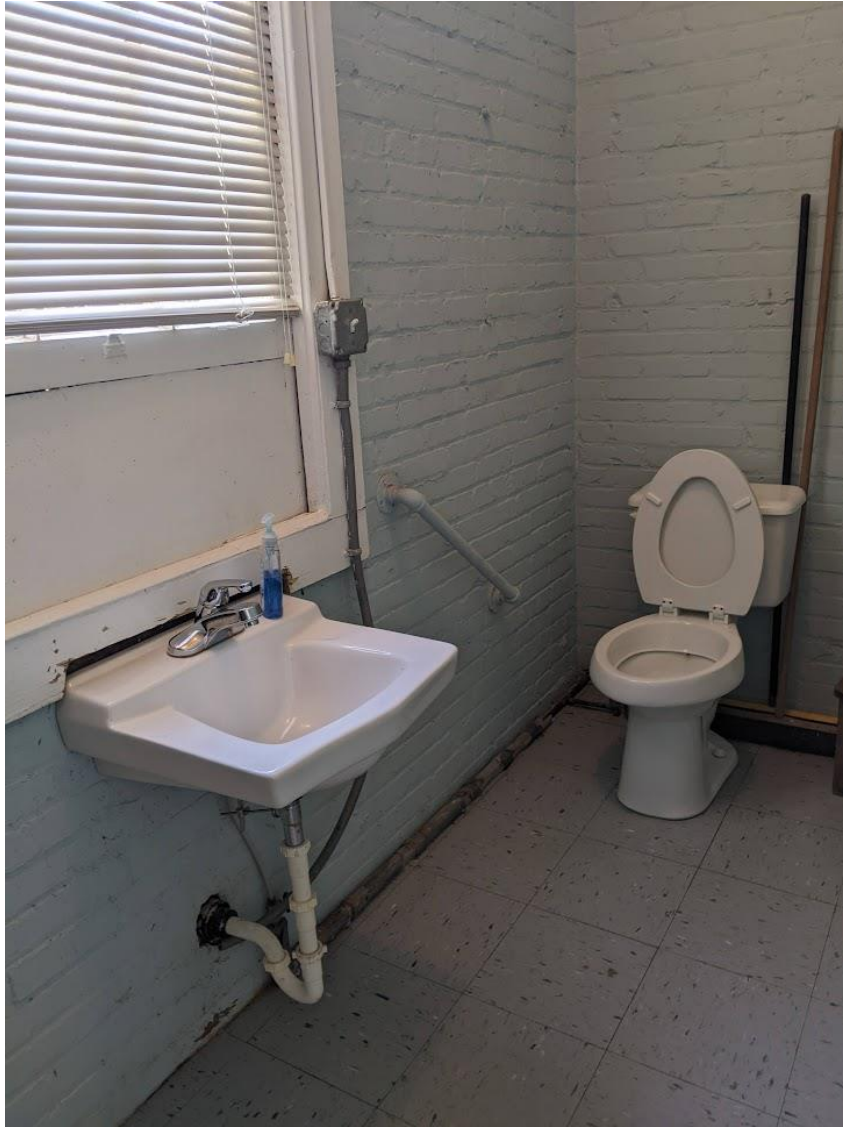
Internal Bathroom #1-Window needing repair. Alternate #3-Add mop sink.
