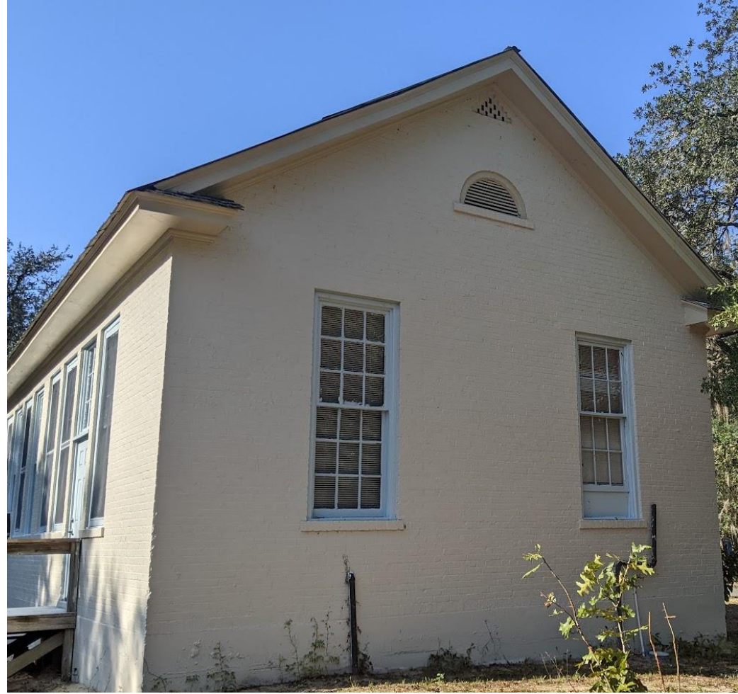
Picture of back of school showing exterior view of two (2) bathroom windows.
