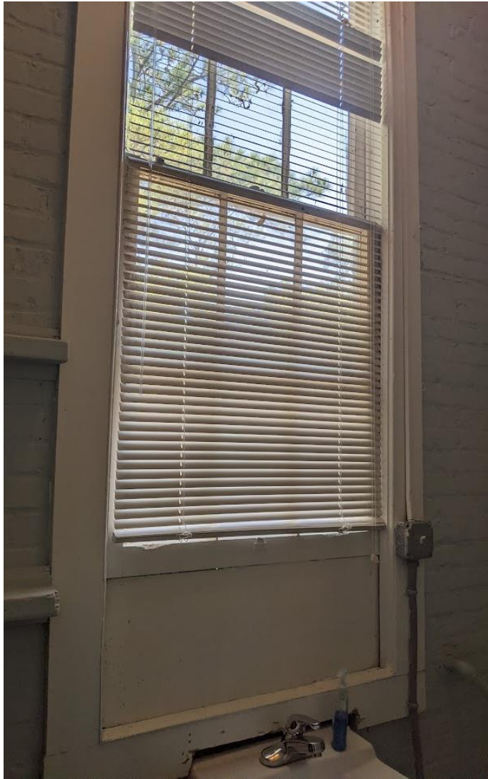
Internal Bathroom #1-Window needing repair-Picture #2.
