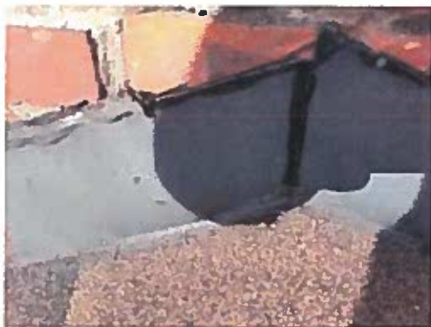
HOMOGENEOUS AREA 07 BRICK MASTIC (BLACK)
