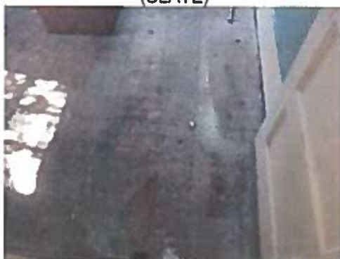
HOMOGENEOUS AREAS 13, 14 9" FLOOR TILE (BEIGE) MASTIC (BLACK)
