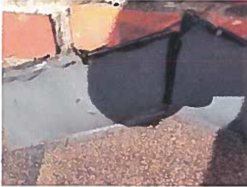
HOMOGENEOUS AREA 07 BRICK MASTIC (BLACK)
