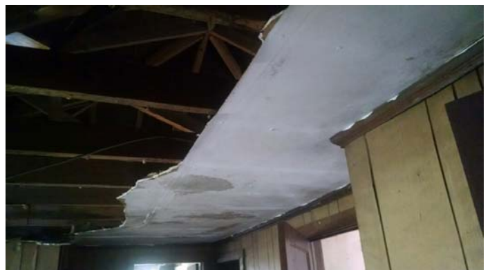
Photo 6 – Typical view of collapsed drywall, joint compound and tape ceiling.
