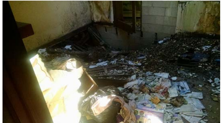
Photo 10 – Typical view of collapsed and unstable flooring in portions of the residence.
