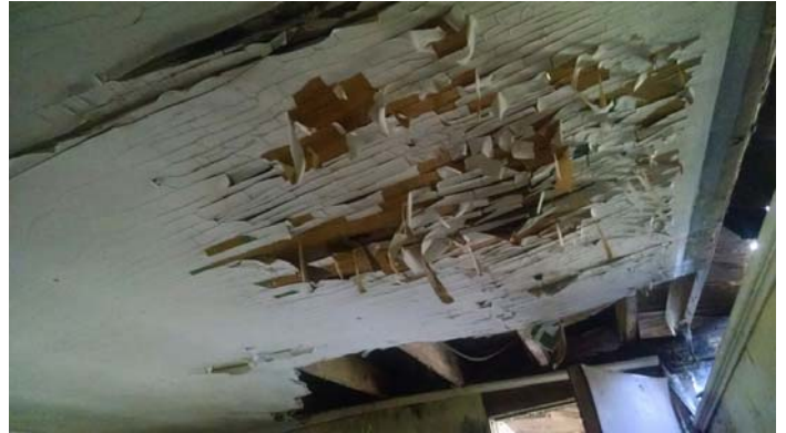
Photo 2 – Drywall, joint compound and tape throughout the ceilings and a quarter of the walls.
