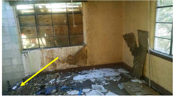
Photo 8 – Typical view of collapsed and unstable flooring in portions of the residence.
