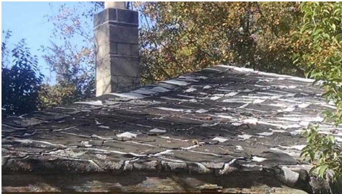
Photo 3 – Roofing shingles and felt on the roof and chimney mastic assumed positive.
