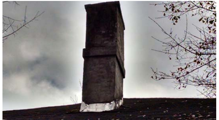
Photo 10 – One chimney with tar assumed.
