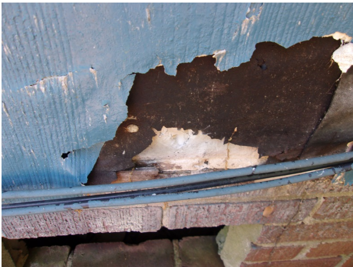
Photo 3 – Cement board siding with felt paper and unfinished drywall beneath.
