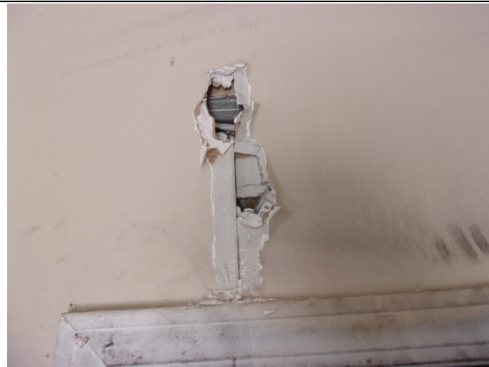
Photo 7 – Top layer of drywall with joint compound & tape in the living room.
