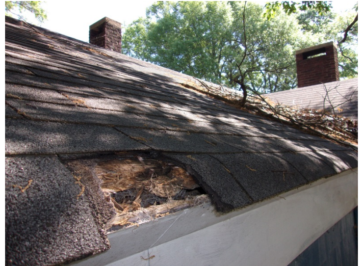
Photo 2 – Roof shingles and no felt & 2 chimneys with mastic/tar assumed positive.
