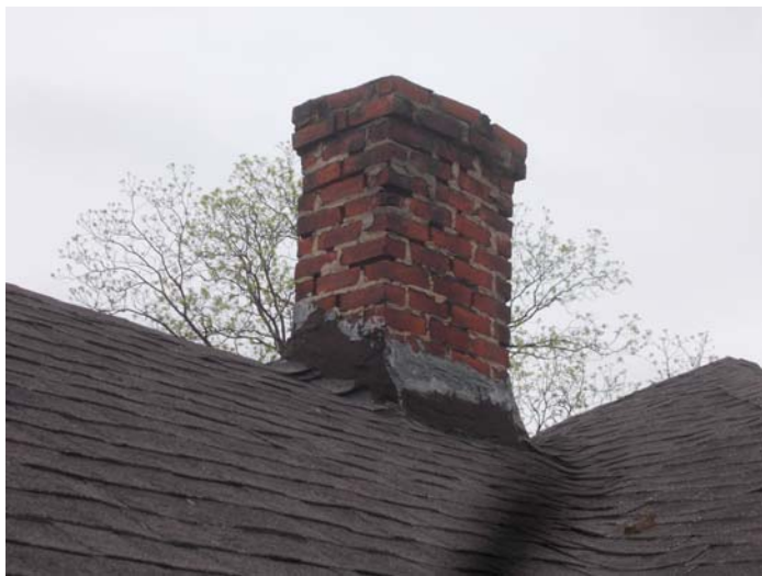
Photo 3 – Two chimneys with tar/mastic assumed positive.
