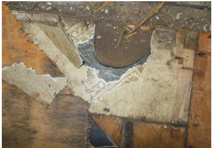
Photo 12 – Three layers of vinyl floor with and with no mastic under wood in kitchen.
