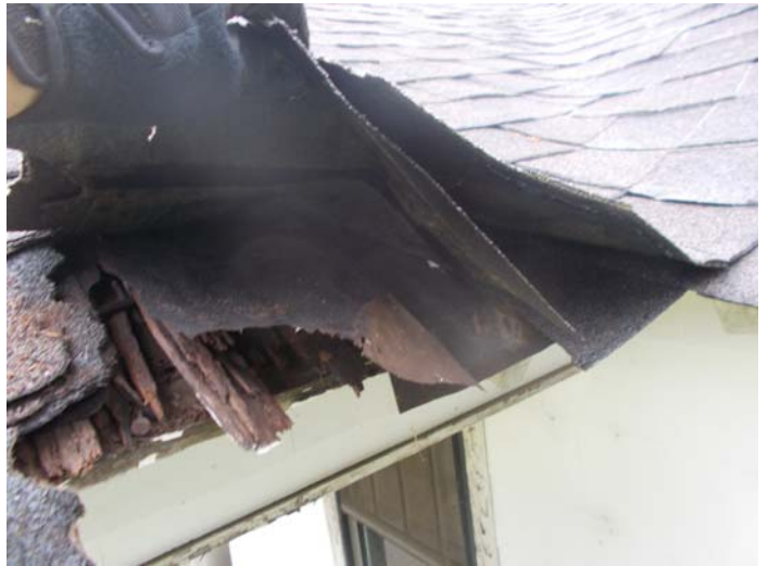
Photo 2 – Roofing shingles (2 layers) and felt (1 layer).
