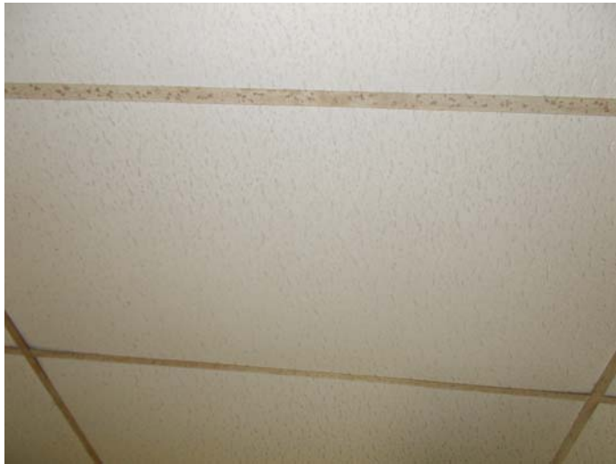
Photo 7 – 2'x4' fissured ceiling tiles throughout grid.
