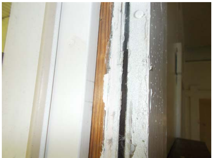
Photo 6 – Caulk on interior door frame.
