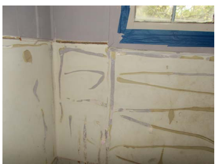
Photo 8 – Wall mastic in shower stall area.
