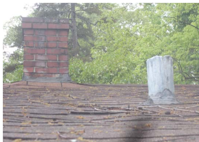
Photo 3 – Chimney and vent penetration with mastic assumed positive.
