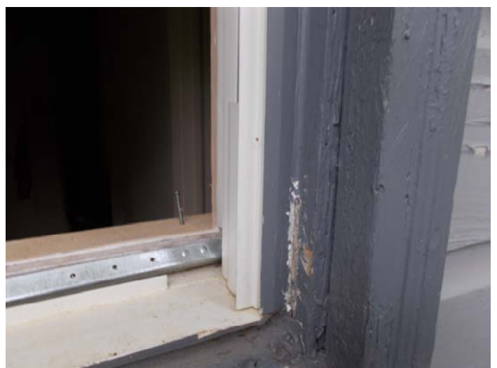
Photo 4 – Caulk on exterior vinyl window.
