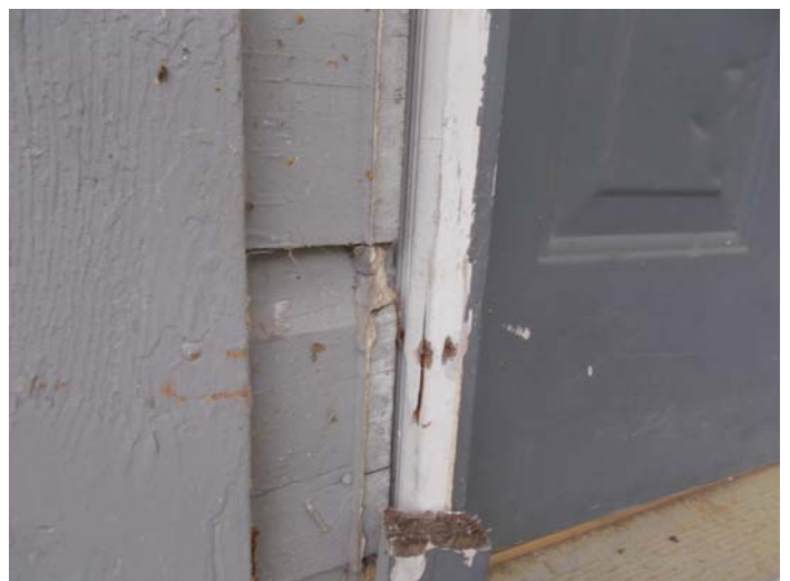
Photo 6 – Caulk on exterior door frame.
