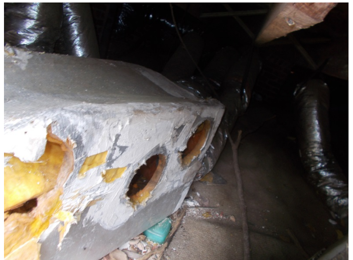
Photo 4 – HVAC mastic in the crawlspace.
