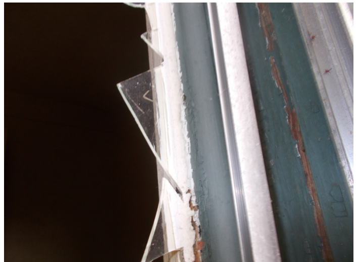
Photo 6 – Inner caulk on window panes.
