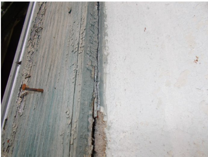
Photo 5 – Outer caulk on exterior windows.
