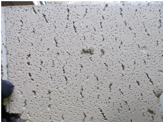
Photo 9 – 2' x 2' fissure ceiling tile in the kitchen.
