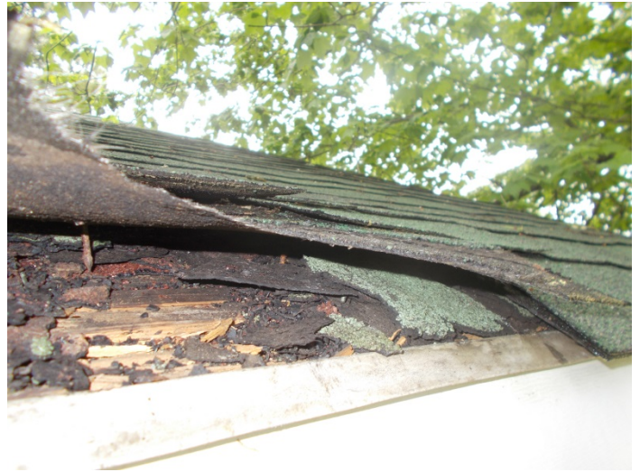
Photo 2 – Roof shingles and no felt.
