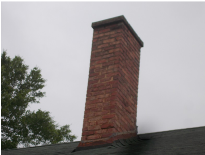
Photo 3 – Typical chimney with mastic assumed positive.
