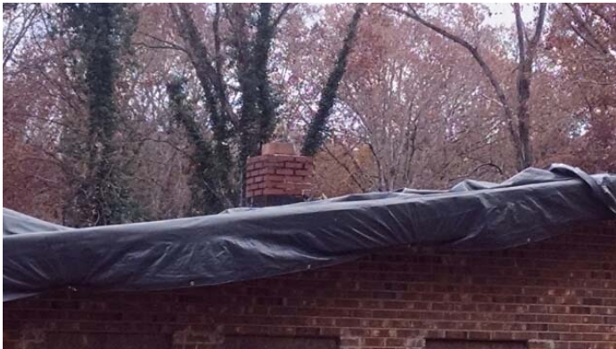
Photo 3 – Chimney with assumed tar.
