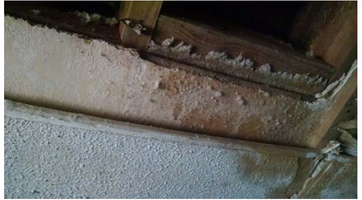
Photo 8 – Ceiling texture, drywall and plaster in kitchen.
