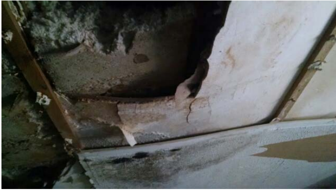
Photo 7 – Ceiling texture, drywall and plaster in kitchen.
