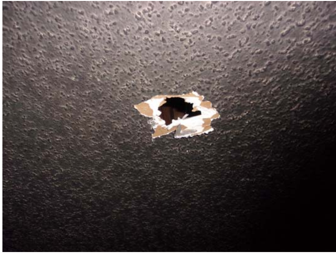
Photo 7 – popcorn ceiling texture throughout
