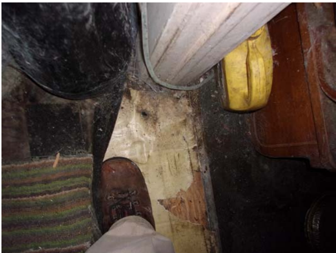
Photo 5 – Tan square pattern roll vinyl floor with no mastic in the bathroom
