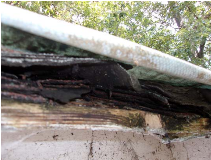
Photo 3 – Roof shingles with no felt
