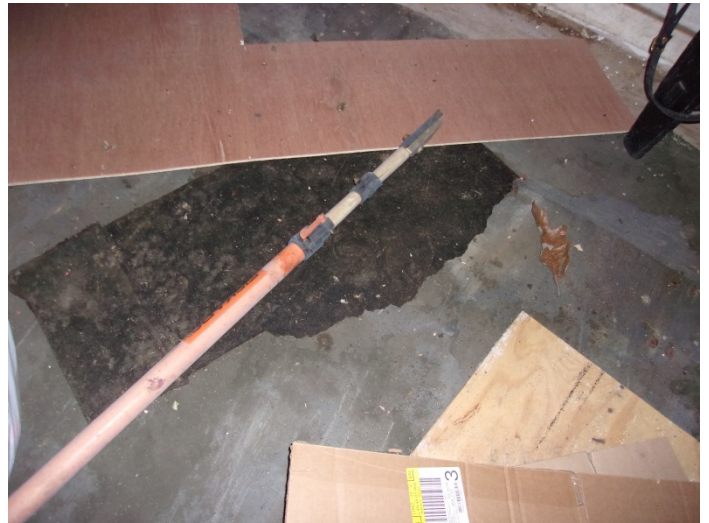
Photo 4 – Black flooring material with no mastic in the front left room off of the kitchen entry door
