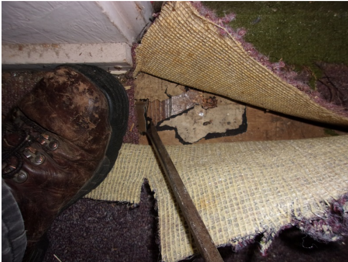
Photo 7 – 2 layers of vinyl floor under carpet in the living room
