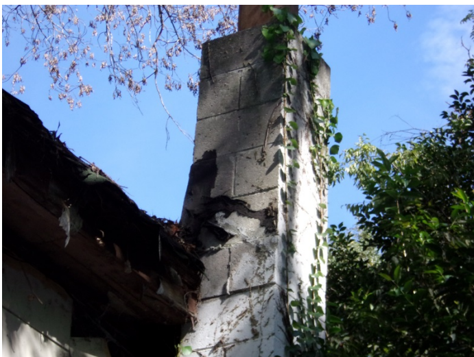
Photo 11 – Tar on chimney at the front of the house
