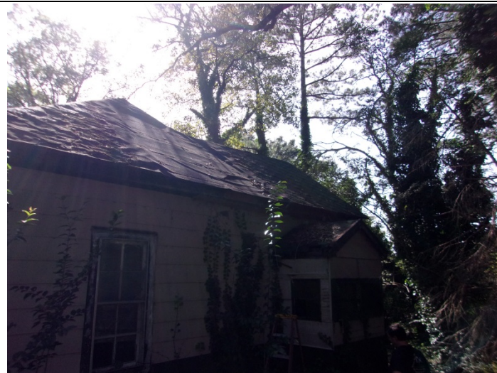
Photo 13 – Red, green & black roof shingles on the main roof of the house
