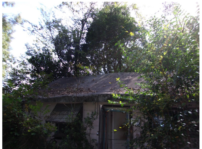
Photo 12 – Roof roll shingles with no felt on the addition of the house
