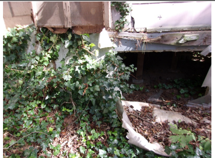
Photo 14 – Tan brick pattern roll vinyl floor with no mastic used as exterior siding
