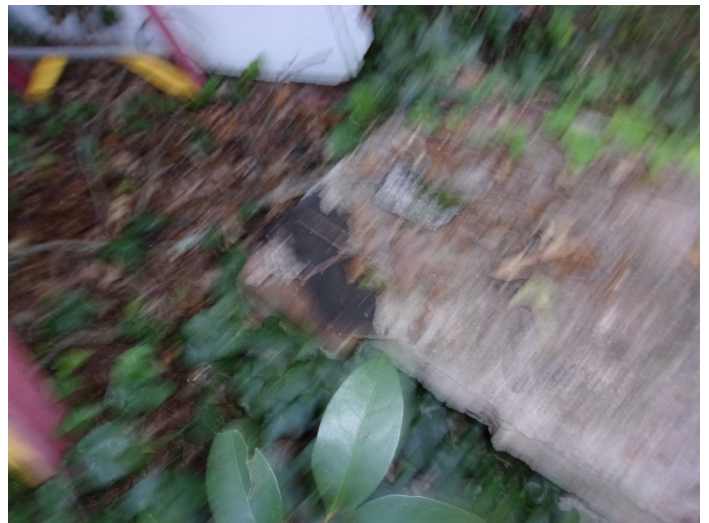
Photo 10 – Tar on chimney on the ground at the back of the house
