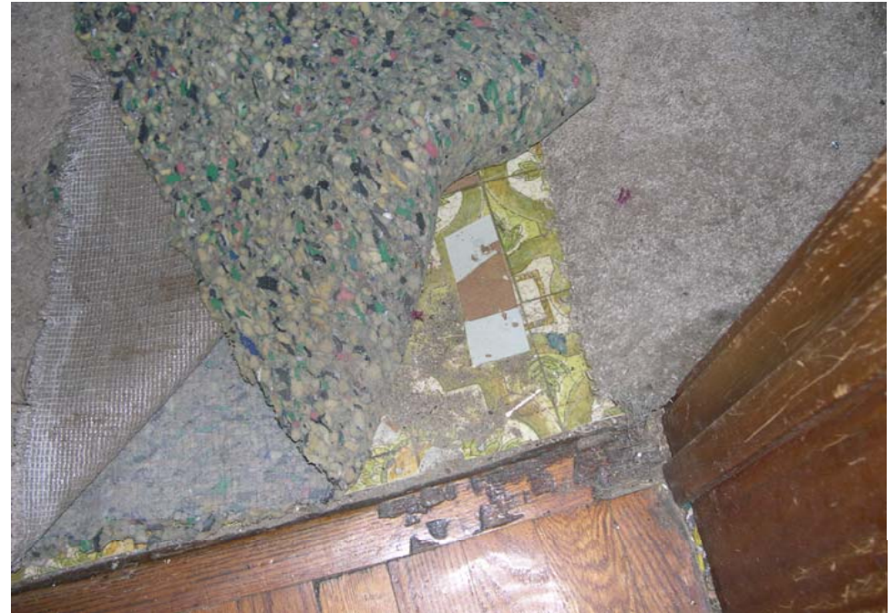
Asbestos floor covering under carpet
