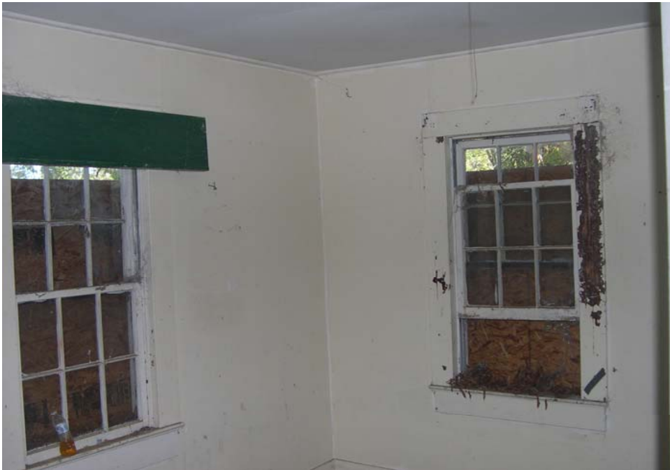
Asbestos joint compound on gypsum board
