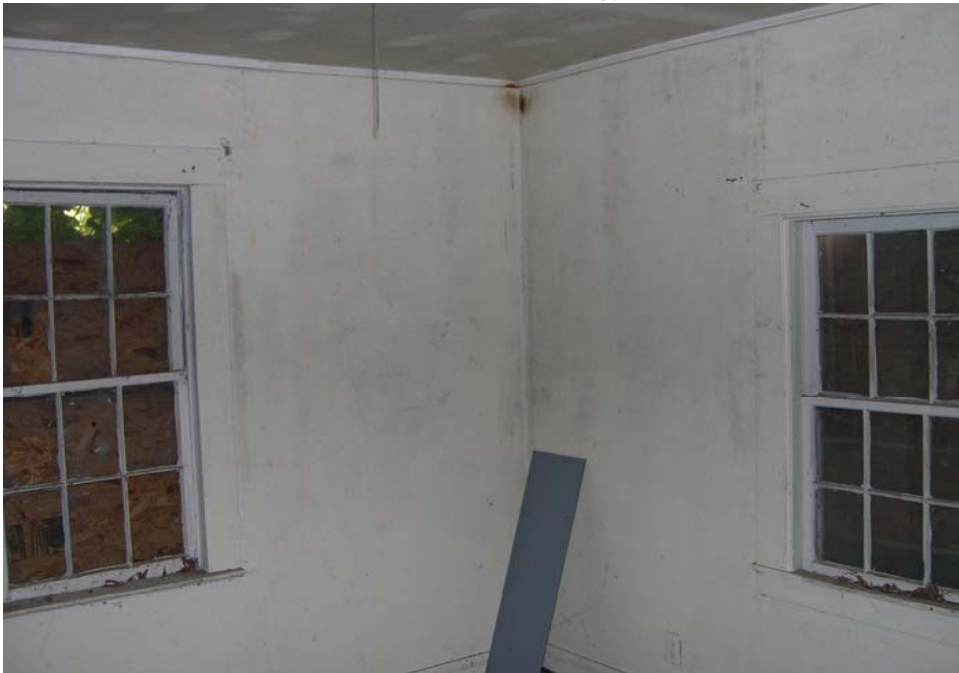
Asbestos joint compound on gypsum board
