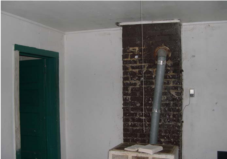
Asbestos joint compound on gypsum board
