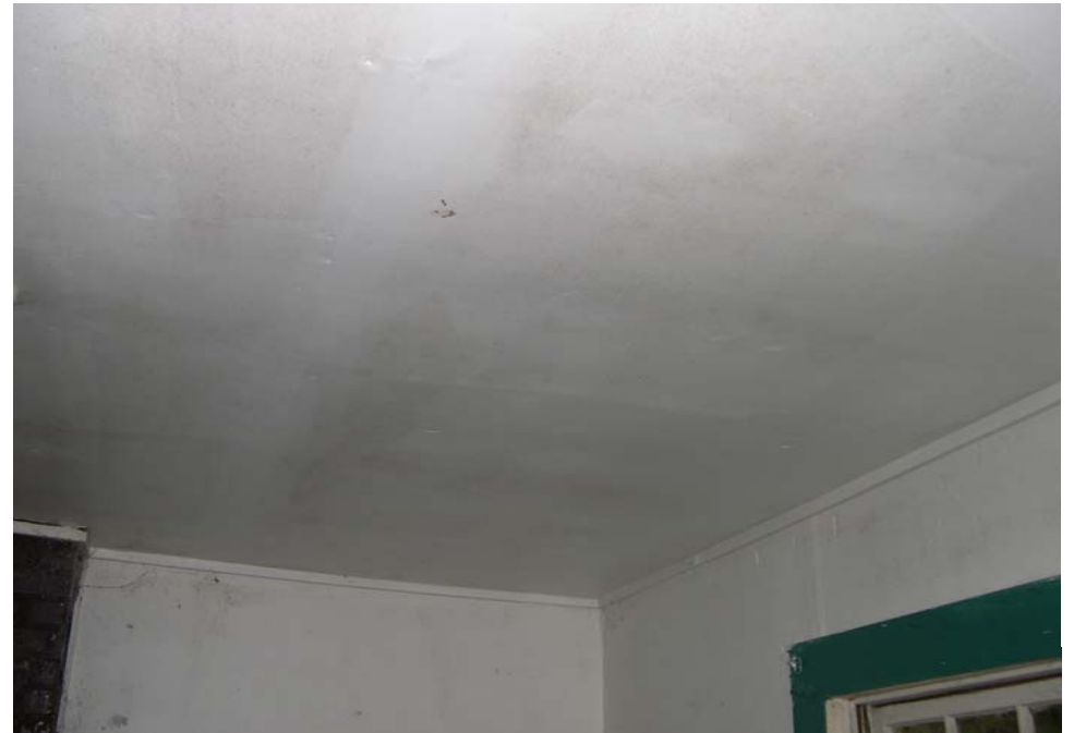
Asbestos joint compound on gypsum board
