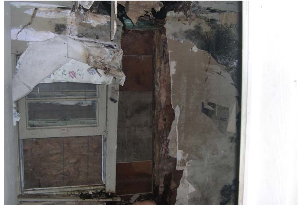
Asbestos joint compound on gypsum board
