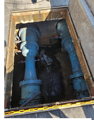
Raw Water Flow Meters at Existing Hicks WPP
