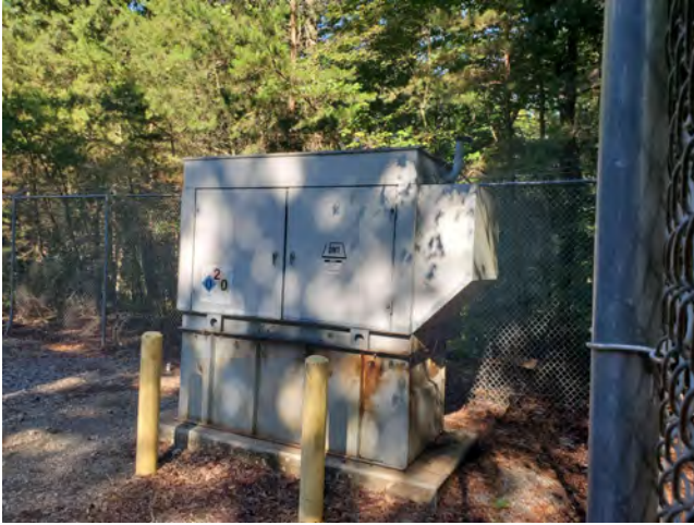
Diesel generator present at the base of cellular tower.
