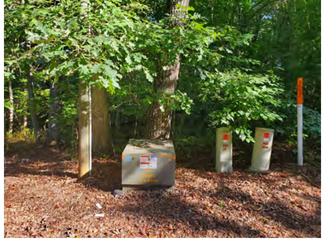
Pad-mounted transformer observed near the base of the cellular tower .
