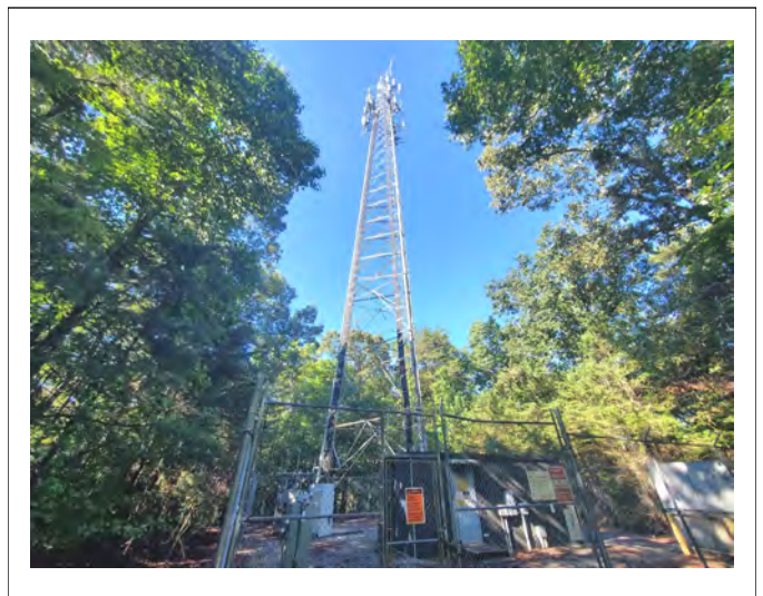
Cellular tower and surrounding fence present in the northern portion of the subject property.
