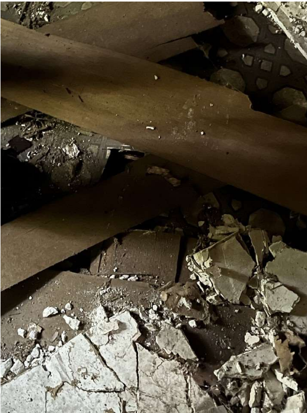
Interior Drywall on Floor
