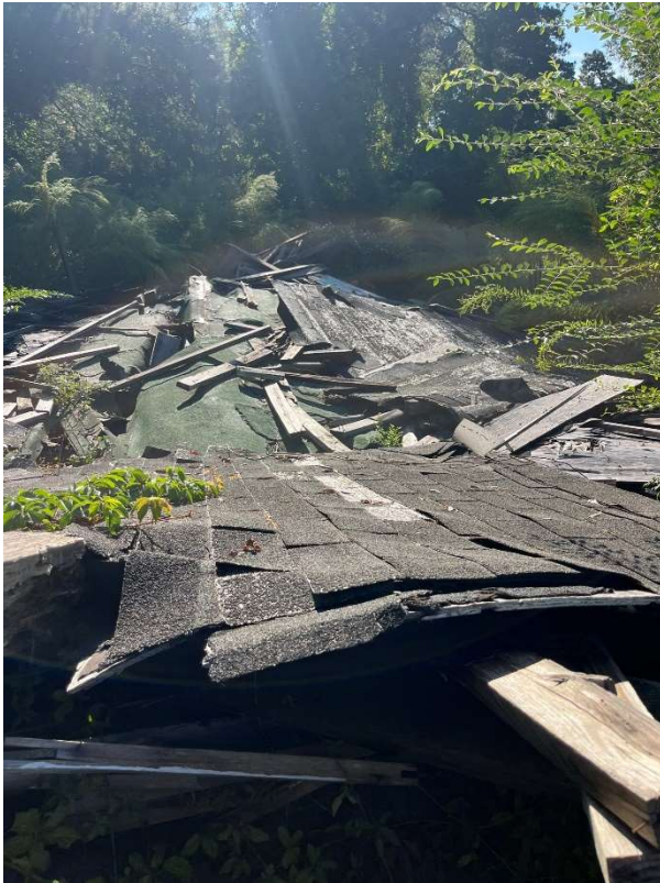
Debris Pile Showing Asphalt Shingles
