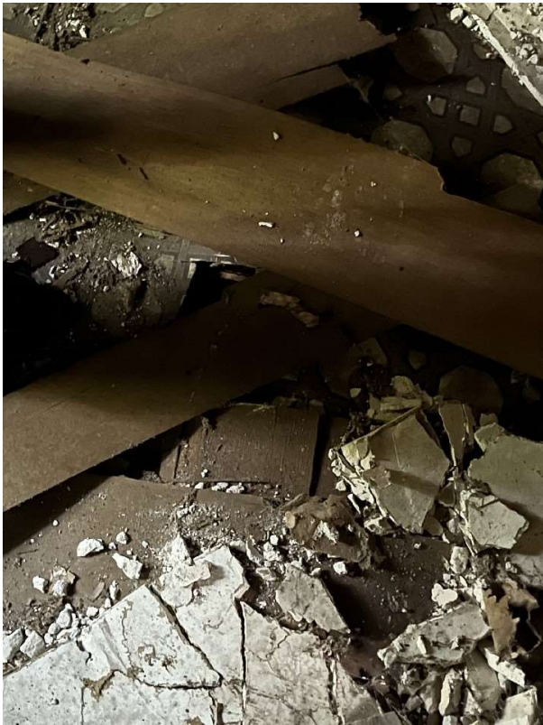
Interior Showing Drywall Debris
