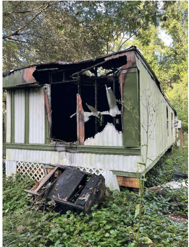
Exterior Right Side Showing Fire Damage
