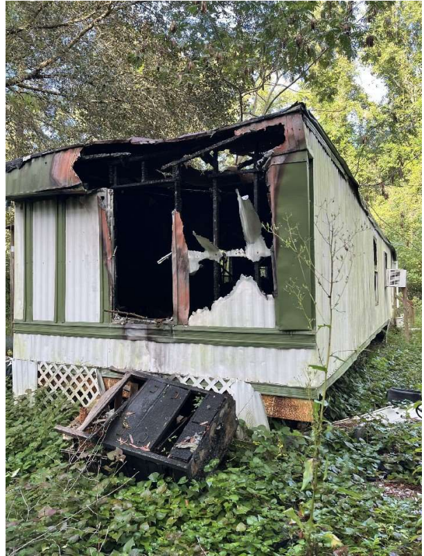
Exterior Right Side Showing Fire Damage
