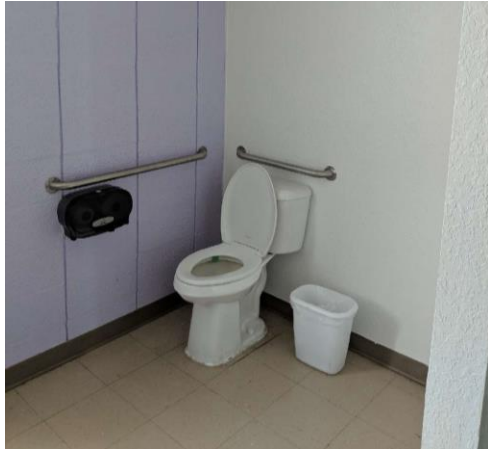
Figure 15: P6 WOMENS RESTROOM – note only one toilet
