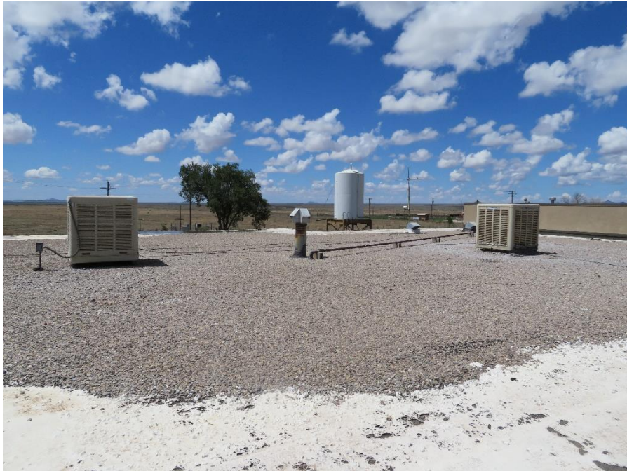
Figure 2: EXISTING COMMERCIAL TERMINAL EVAPORATIVE COOLERS
