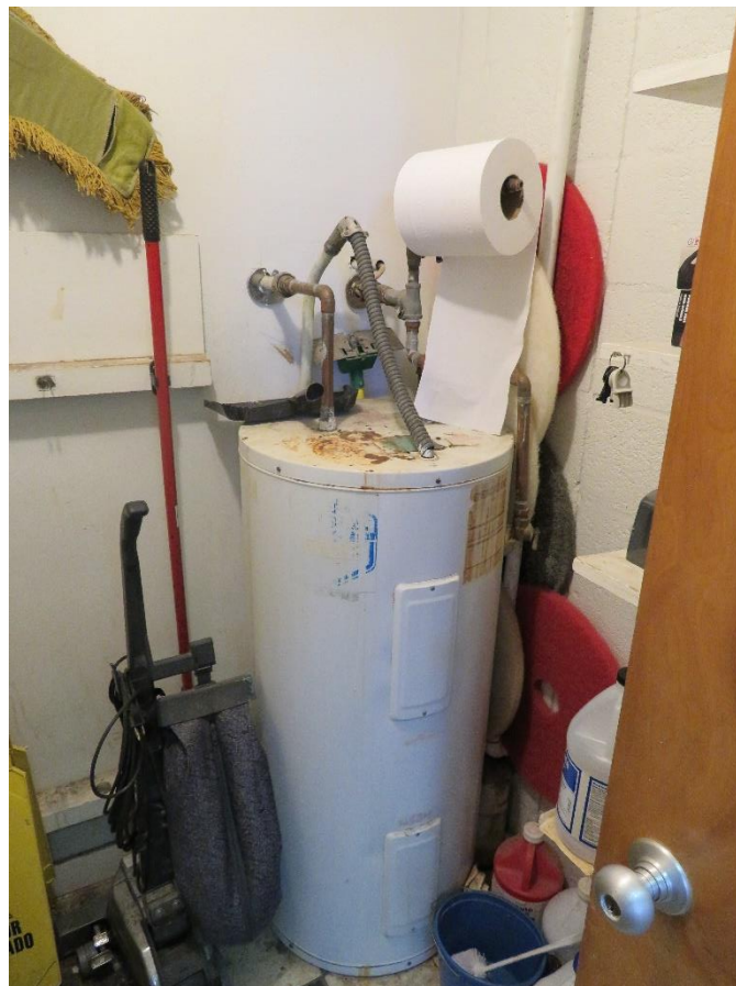
Figure 4: EXISTING COMMERCIAL TERMINAL WATER HEATER
