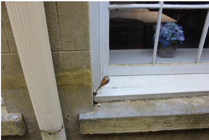
Figure 139: The sill is deteriorated on the left hand side.
