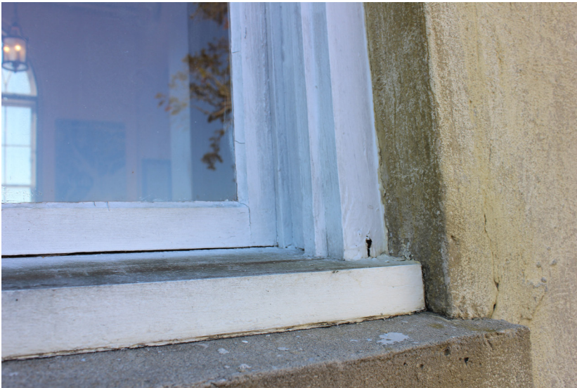
Figure 92: Ferrous fasteners within the window are actively corroding.
