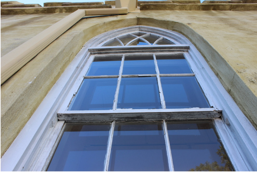
Figure 95: The upper sash is damaged and is cracking along the stiles.
