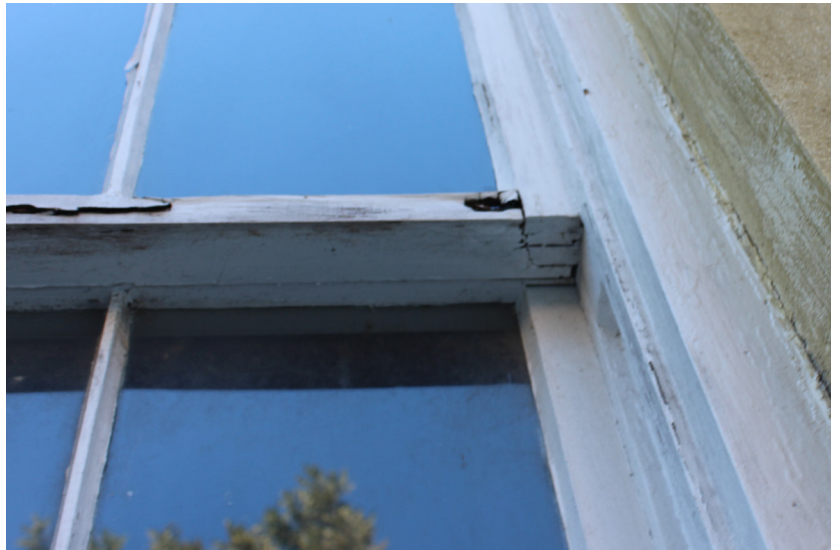
Figure 8: Common failures include deterioration at the meeting rail and the bottom rail of the lower sashes.
