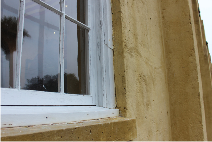
Figure 23: The casing on the lower right hand side has been repaired with a dutchman. The dutchman is now releasing from the casing.
