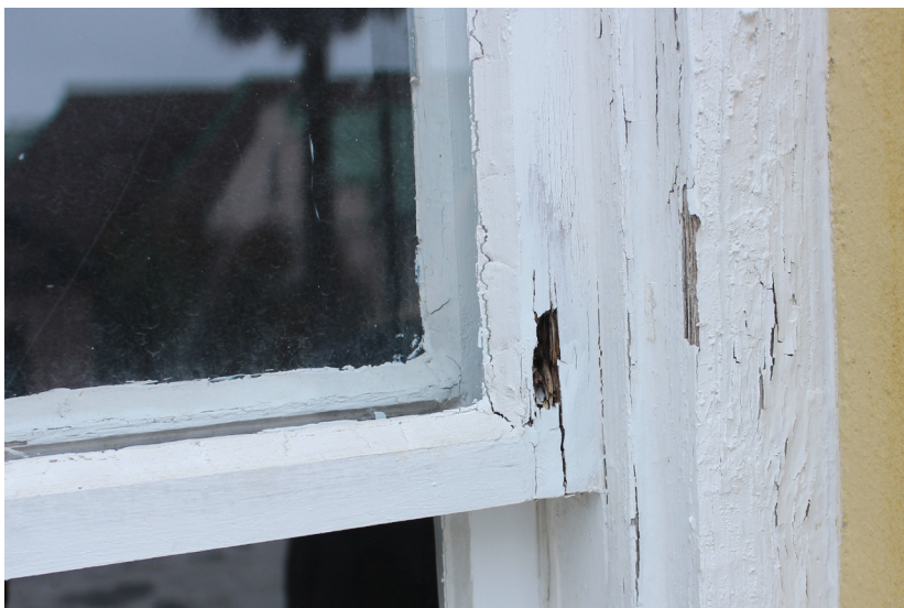
Figure 13: The upper sash is deteriorated at the intersection of the right stile and bottom rail.
