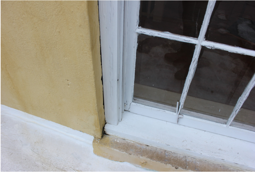
Figure 52: The lower sash is deteriorated on the right hand side.
