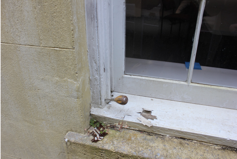
Figure 134: The bottom of the casing on the left hand side is deteriorated.
