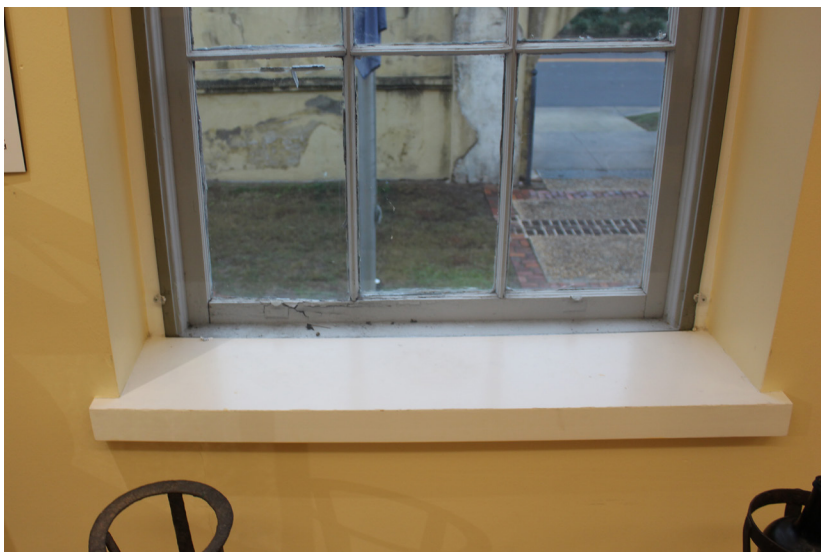
Figure 37: The lower sash is completely deteriorated and visible on the interior of the window.
