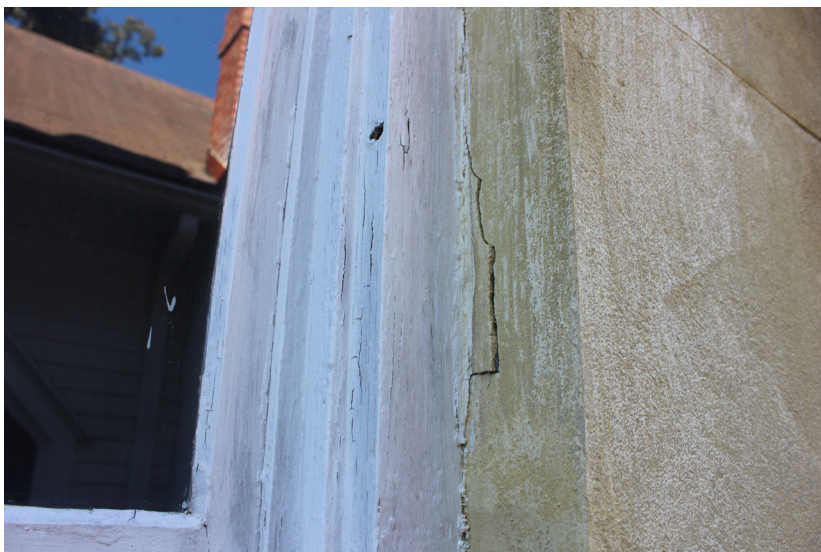
Figure 129: Detail of hole within the casing to secure plywood used for hurricane protection.
