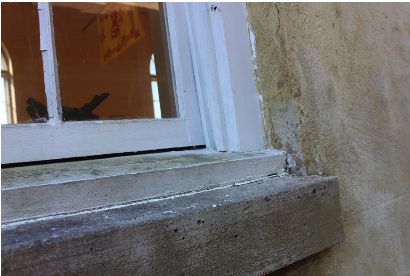
Figure 104: A gap is present between the lower sash and the sill. Biogrowth is present on the sill.
