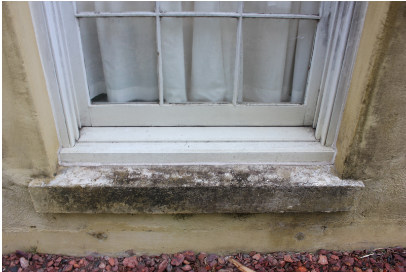
Figure 71: Biogrowth is present throughout the window.
