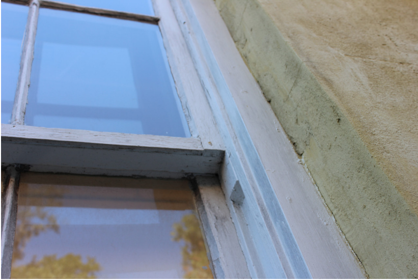
Figure 115: There is moderate separation of the joints within this window.
