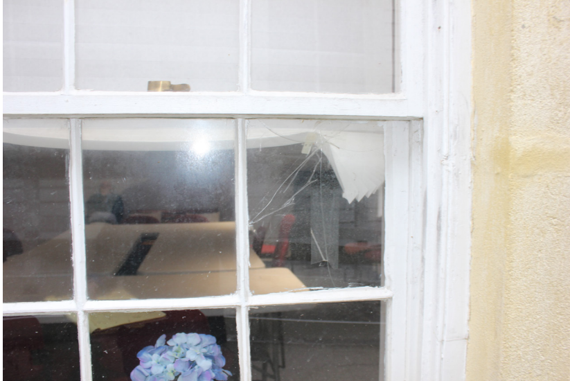
Figure 138: Detail of broken glass.
