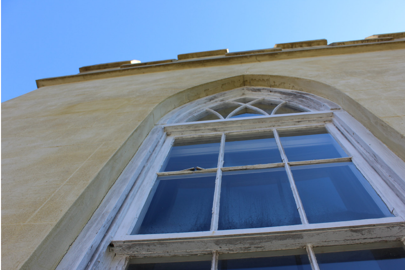
Figure 142: A muntin is broken on the upper sash. Select areas of the sill are deteriorated.
