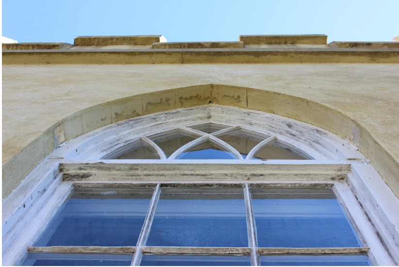
Figure 146: Biogrowth is present on all wooden elements.
