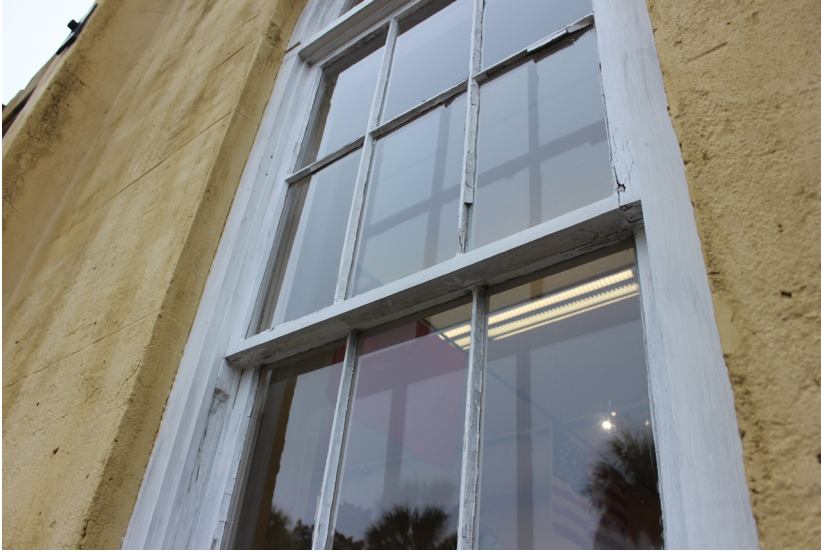
Figure 31: The right stile of the upper sash is deteriorated. A broken muntin is also visible within the upper sash.
