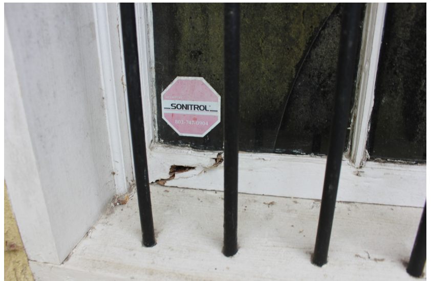
Figure 9: Detail of deterioration on a fixed casement window.
