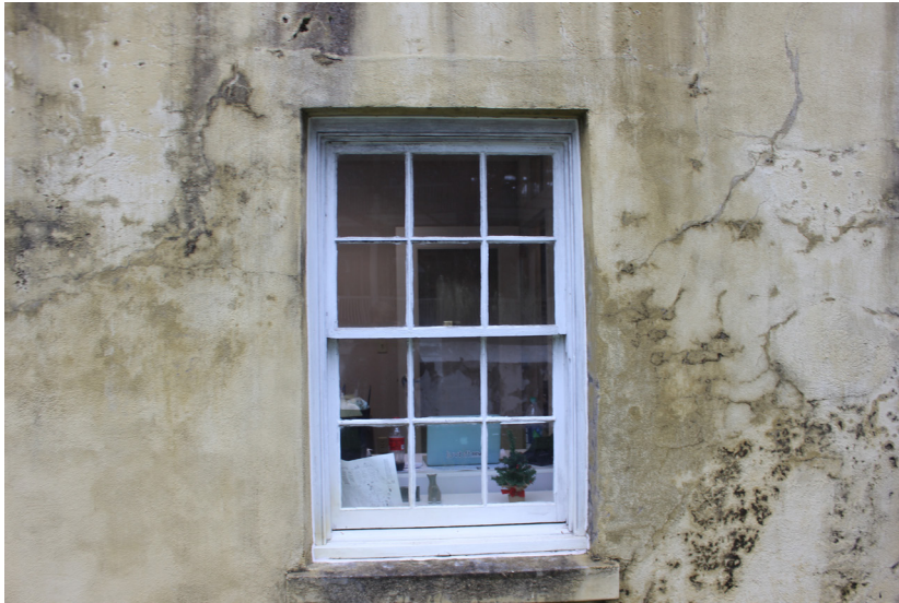
Figure 158: Biogrowth is present throughout the masonry opening.
