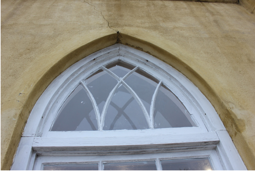
Figure 51: The transom casing is beginning to separate at the joints. The glass is in good condition.
