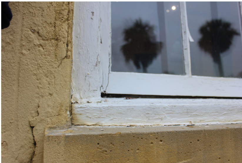
Figure 20: The left side of the window has been repaired with a composite material. The casing may be damaged beneath this repair.
