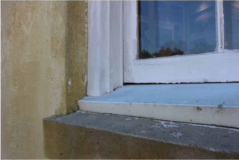
Figure 88: The sill is in good condition. There is moderate separation of the joints within the wooden window.
