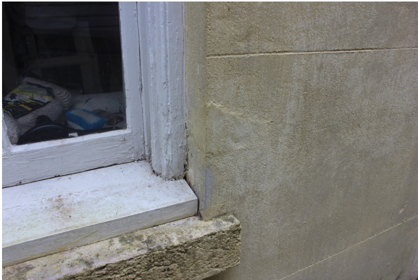
Figure 132: Detail of inappropriate repairs.
