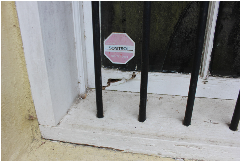
Figure 84: The window is heavily deteriorated at the bottom. The pane of glass is broken at the location.
