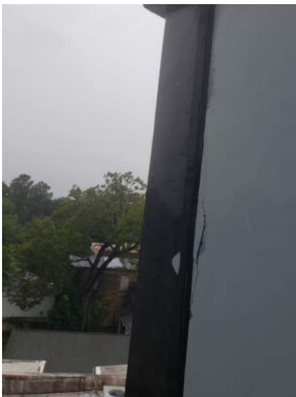
PHOTO 40: SPALLED CONCRETE COVER OVER PANEL JOINT
