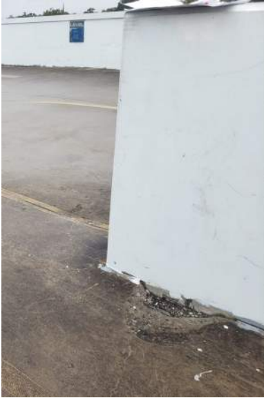
PHOTO 9: CONCRETE TOPPING DAMAGE AT UPPER LEVEL
