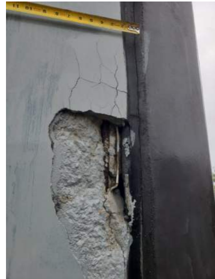
PHOTO 39: CLOSE UP OF SPALLED CONCRETE AND CORRODED REINFORCING
