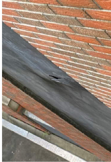
PHOTO 21: ISOLATED SPALLING ON EAST WALL (FROM ABOVE)
