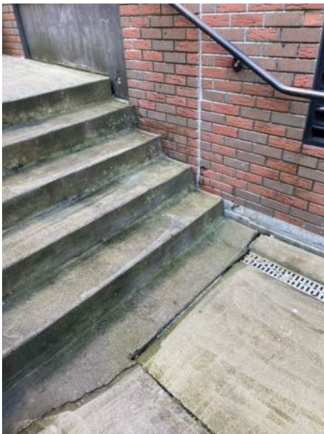
PHOTO 28: DAMAGED BRICK VENEER
