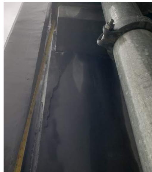
PHOTO 41: SPALLED CONCRETE COVER OVER PANEL JOINT BELOW UPPER LANDING
