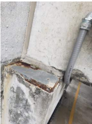
PHOTO 19: CORRODED BEAM BEARING PLATE
