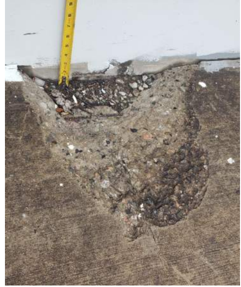
PHOTO 10: CLOSE UP OF CONCRETE TOPPING DAMAGE AT UPPER LEVEL
