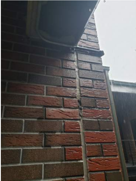
PHOTO 26: DETERIORATED CAULK IN WALL PANEL JOINTS
