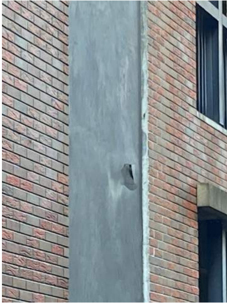
PHOTO 20: ISOLATED SPALLING ON EAST WALL
