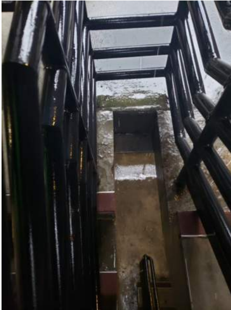
PHOTO 22: RAINWATER RUNOFF BETWEEN STAIR FLIGHTS
