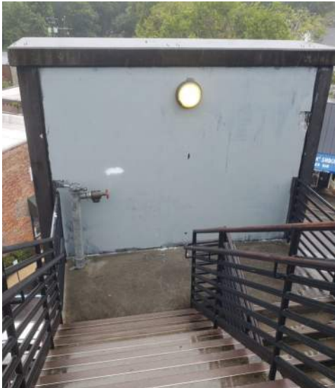
PHOTO 38: SPALLED CONCRETE COVER OVER PANEL JOINT
