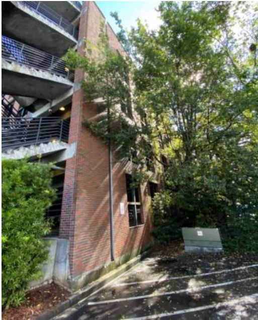
PHOTO 1: VEGETATION AGAINST THE SOUTH EXTERIOR WALL
