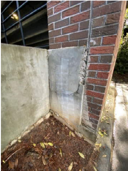
PHOTO 55: CRACK THROUGH EXTERIOR BRICK VENEER
