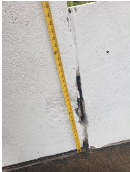
PHOTO 11: SPALLED UPPER LEVEL PANEL CONNECTION
