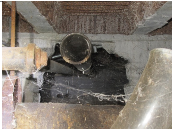
Photograph #3: Access point/entrance to the crawlspace area pictured in Figure 1 above with the blue outline & black X. The pictured (open) pipe exits below the Library/Media Center slab/foundation and appears active.
