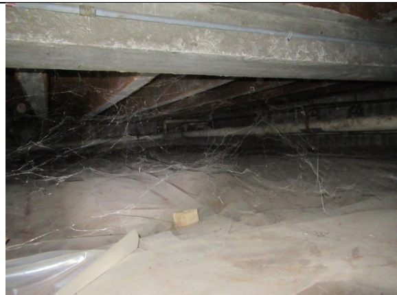
Photograph #4: View towards the crawlspace area below Room 110, at the adjacent Boy's restroom. (See section 19.8 above)
