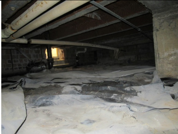
Photograph #1: View towards the crawlspace entrance below Room 104 and the Boy's restroom.
