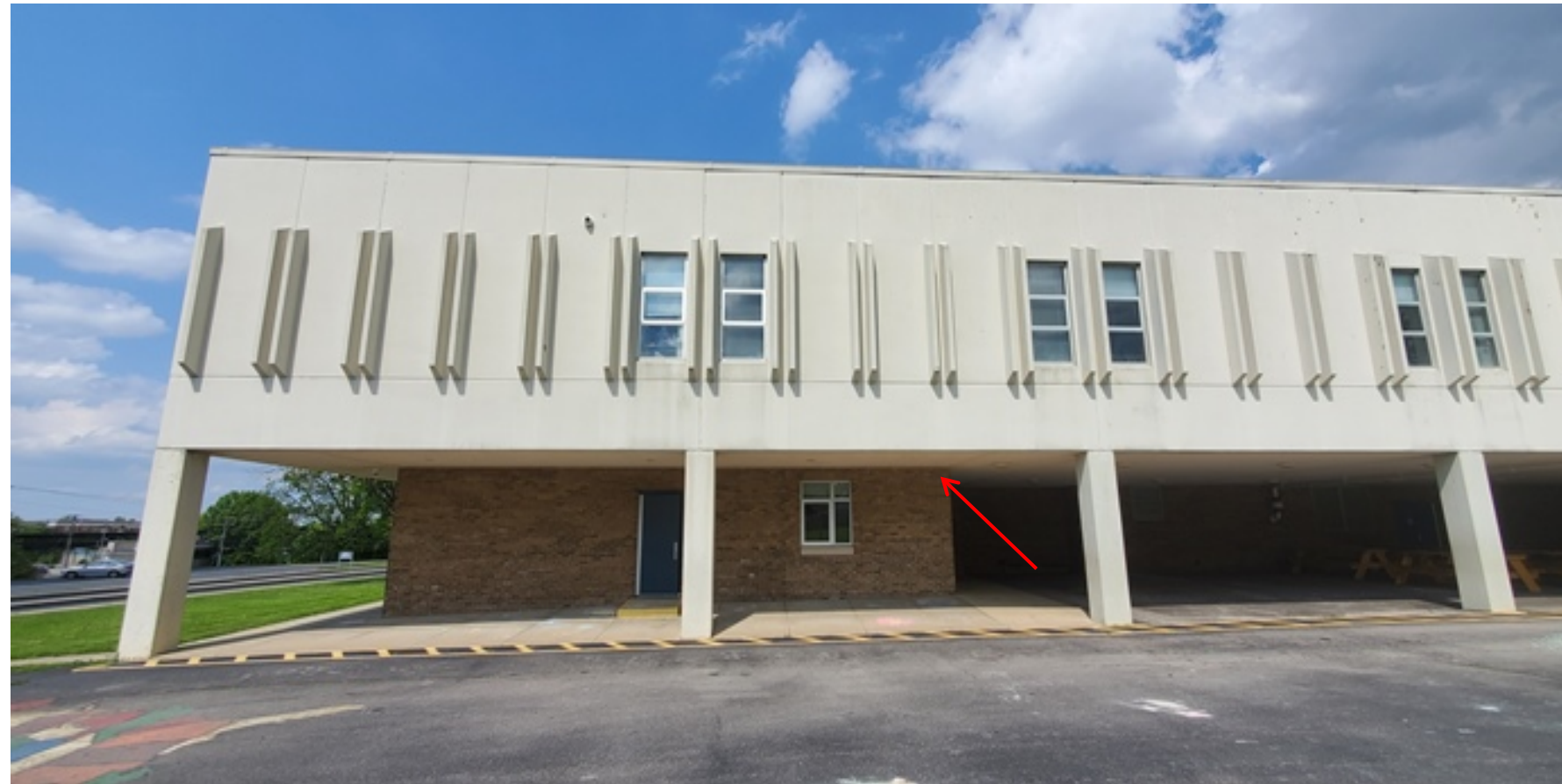
Figure 2: Possible exhaust location/pathway out of the Conference Room. (No system and/or piping shall be present on the front of the building)
