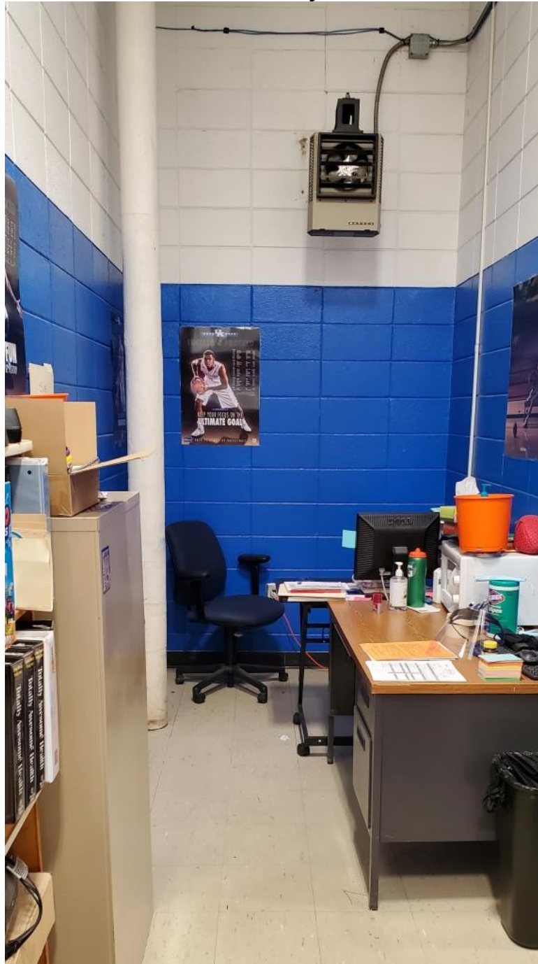
Figure 2: View of Gym Office (Room #512B) (Roof drain penetrates the floor)
