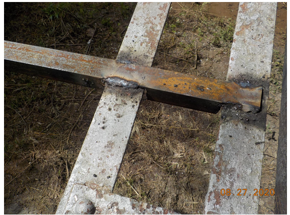
Temporary scaffold support braces welded to the bottom chord on both sides.
