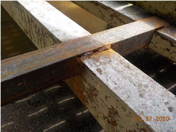
Temporary scaffold support braces welded to the bottom chord on both sides.
