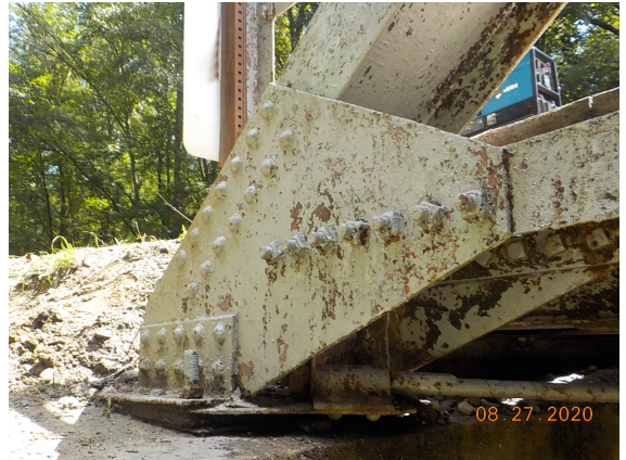
Abutment 1, right exterior gusset plate has minor to moderate rust and corrosion.
