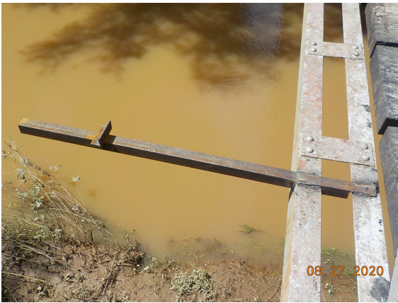
Temporary scaffold support braces welded to the bottom chord on both sides.
