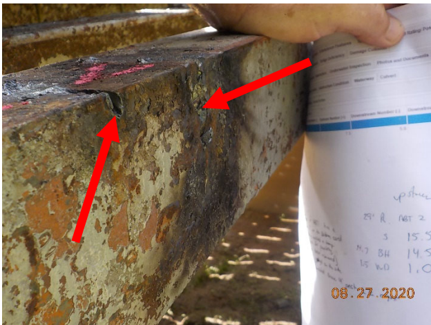
Gouge in Angle Iron Bracing
