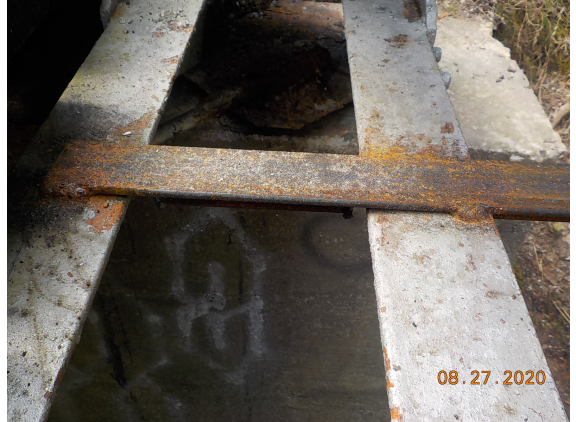
Temporary scaffold support braces welded to the bottom chord on both sides.
