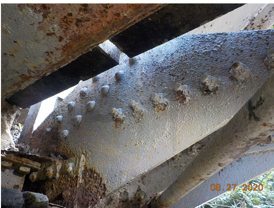
Abutment 1, left interior gusset plate has moderate rust and corrosion with section loss; from 0.188" to 0.25" remaining and needs to be repaired.
