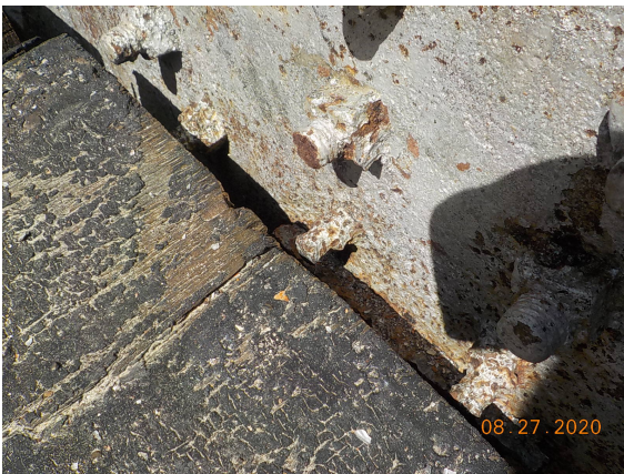
Lower gusset plate nuts rusted away. L 6 right pictured; others similar.
