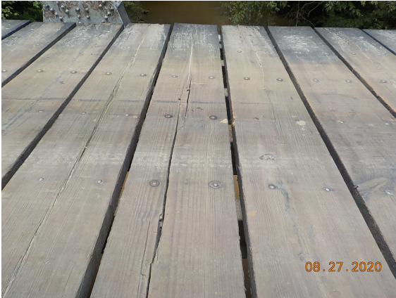
Deck board split
