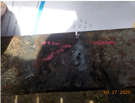
Right bottom chord, 6.0' forward of abutment 1; temporary brace removed leaving a crack/notch on the top of angle and a gouge on the exterior face.
