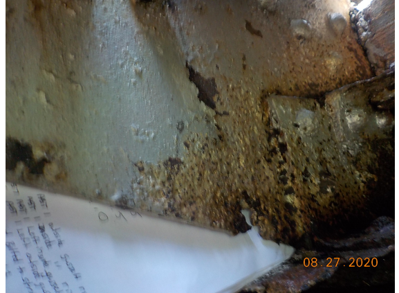
Abutment 2, left interior gusset plate has severe corrosion/section loss with some 1/16" to 1/8" dia. holes. 0.12" remaining in this area. 9/01/2010: Small holes now make one larger hole 1.5" long x
