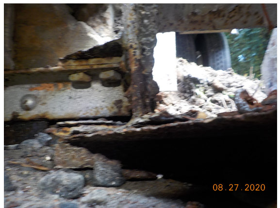
Abutment 1, left interior gusset plate has moderate rust and corrosion with section loss; from 0.188" to 0.25" remaining and needs to be repaired.
