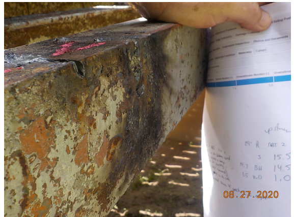
Right bottom chord, 6.0' forward of abutment 1; temporary brace removed leaving a crack/notch on the top of angle and a gouge on the exterior face.
