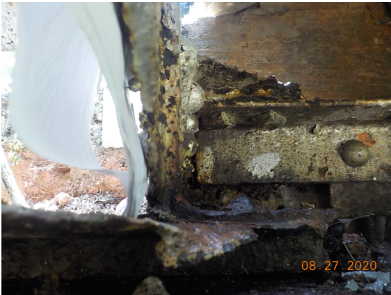
Abutment 2, left interior gusset plate has severe corrosion/section loss with some 1/16" to 1/8" dia. holes. 0.12" remaining in this area. 9/01/2010: Small holes now make one larger hole 1.5" long x
