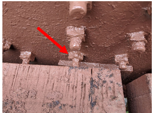
Example of Typical Damaged Bolt
