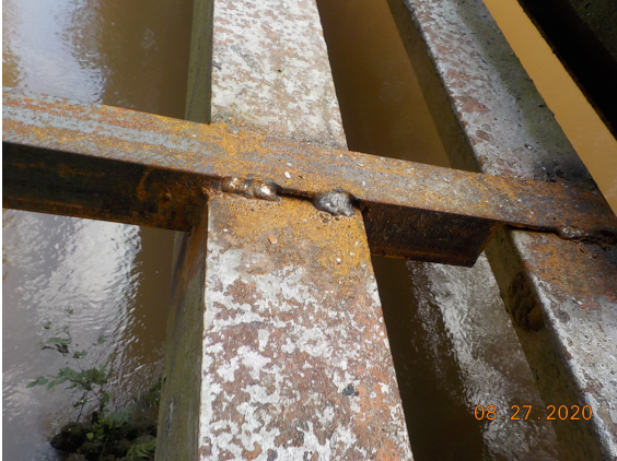
Temporary scaffold support braces welded to the bottom chord on both sides.
