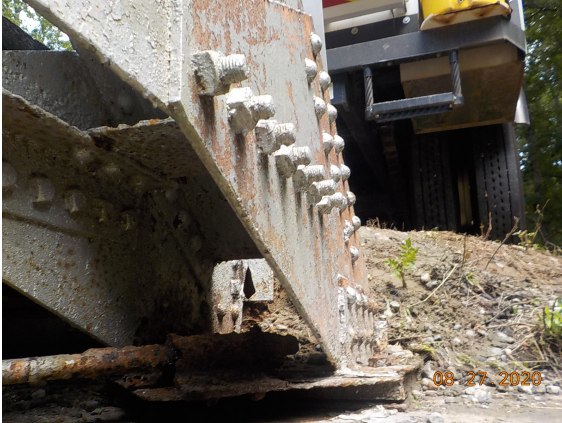
Abutment 1, left exterior gusset plate has moderate rust and corrosion with section loss up to 0.0625"
