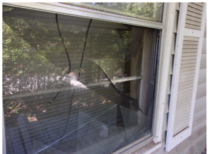
Photo 12 – wooden window glazing.
