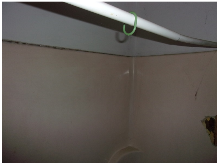
Photo 4 – Shower stall caulk in the bathroom.
