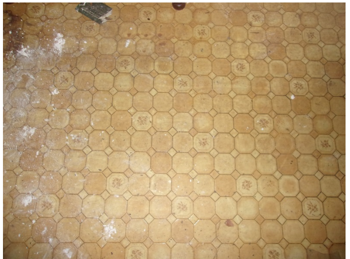
Photo 6 – Yellow octagon pattern vinyl flooring with mastic in the living room (patch).
