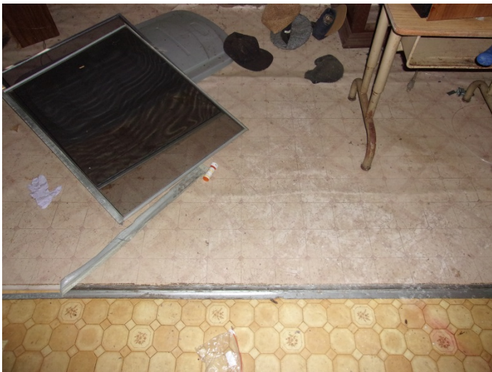
Photo 5 – Grey square pattern vinyl flooring with no mastic in the living room (patch).
