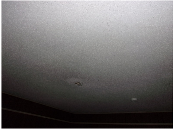
Photo 2 – Popcorn ceiling texture throughout.
