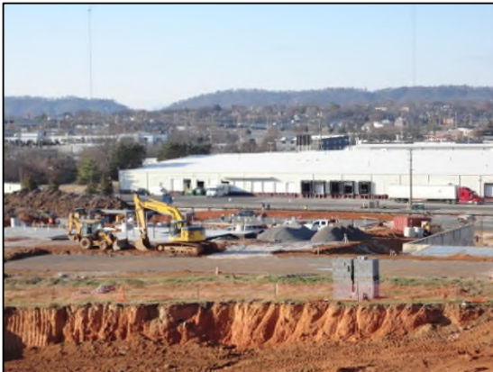
Austin Homes Phase I (Bell Street Flats) under construction to the north.
