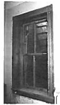
Following the relatively simple repairs, the window is weathertight, like new in appearance, and serviceable for many years to come. Photo: NPS files.
