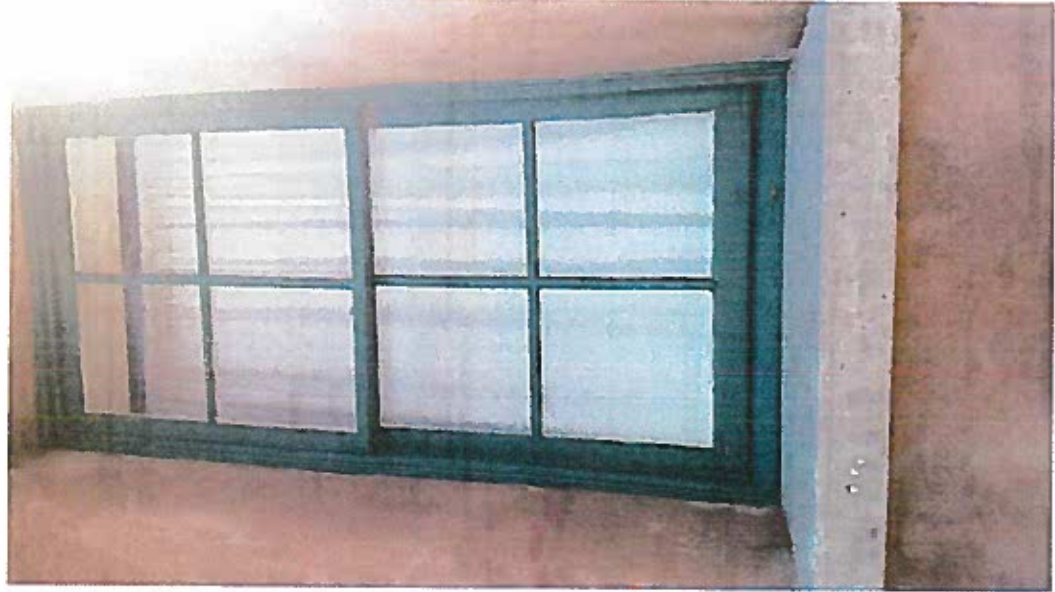
Window 9 – Level A work This east facing window is in very good condition, different from other windows on this elevation
